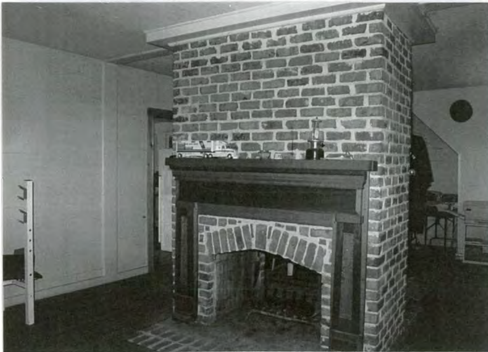
21. Interior view of first floor of rear wing showing brick fireplace and removed interior wall
