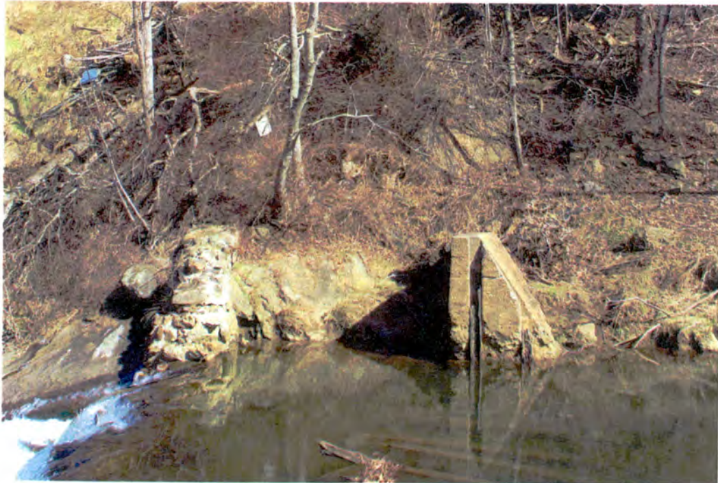
Photograph 43: North bank of the Little River showing remnants of dam wall and poured concrete wall.
