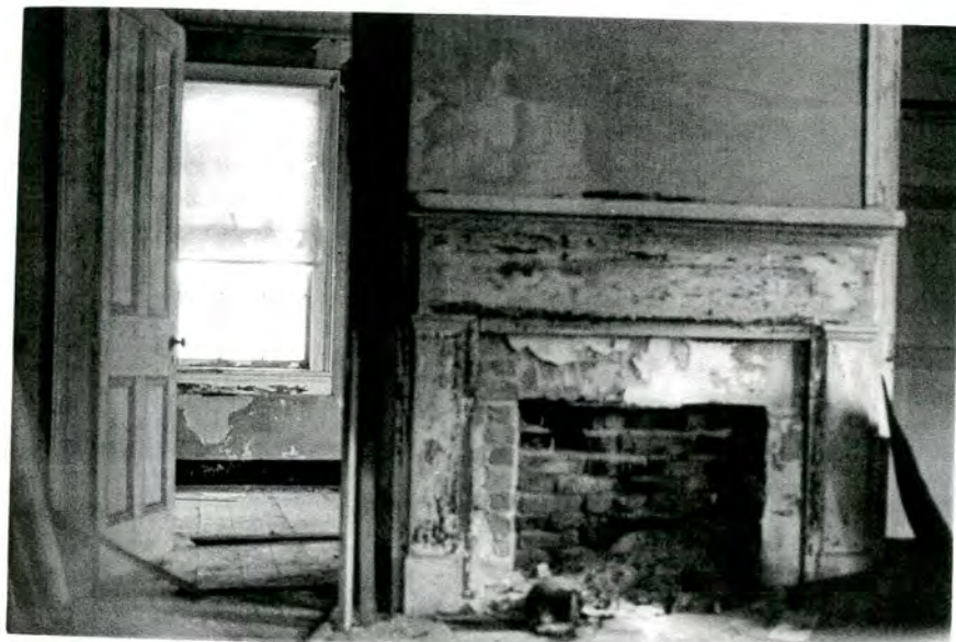
Plate 40. Amos L. Simmons, Jr. House, Interior, Mantel and Doorway, South Rear Room of Main Block.
