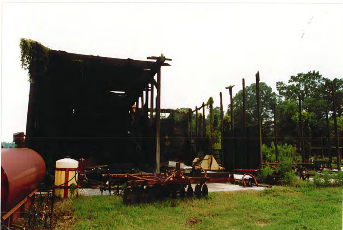
Figure 50. Ruinous machine shed
