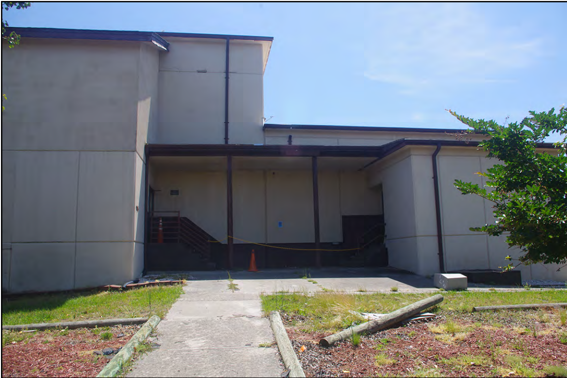
PLATE 26: Detail of West Elevation, Building 116 (NH2664), New Hanover County, North Carolina, Looking East
