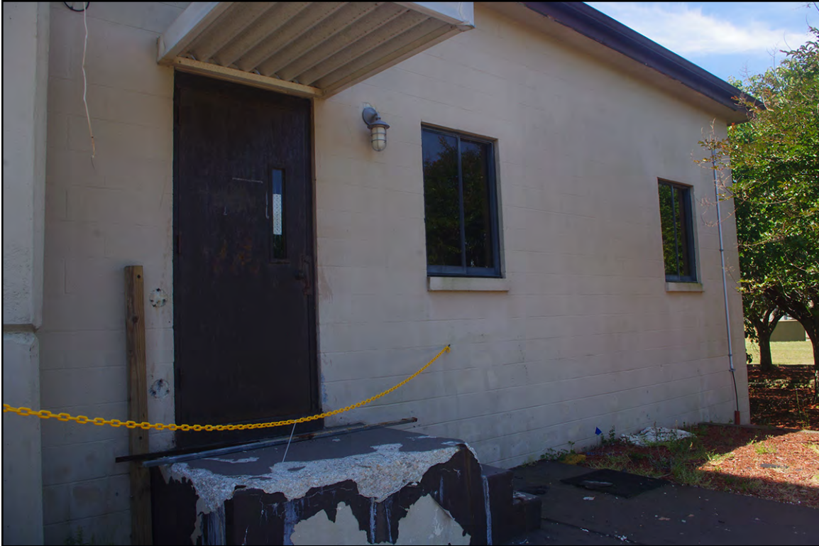
PLATE 20: One-story Addition Extending off North Elevation of Building 116 (NH2664), New Hanover County, North Carolina, Looking Southwest
