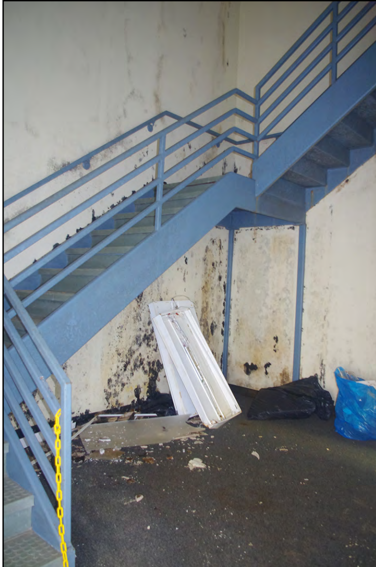
PLATE 28: Detail of Interior Stairwell, Building 116 (NH2664), New Hanover County, North Carolina, Looking Northeast
