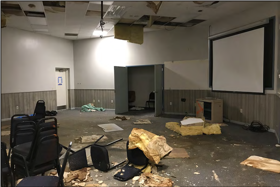
PLATE 29: Interior of Classroom, Building 116 (NH2664), New Hanover County, North Carolina, Looking North
