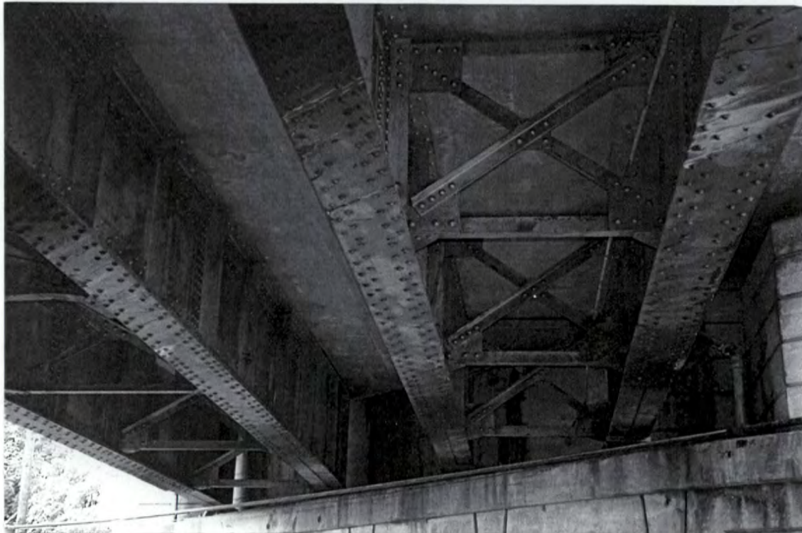
Plate 12: Highland Avenue Southern Railway Bridge – plate girders and cross frames looking west
