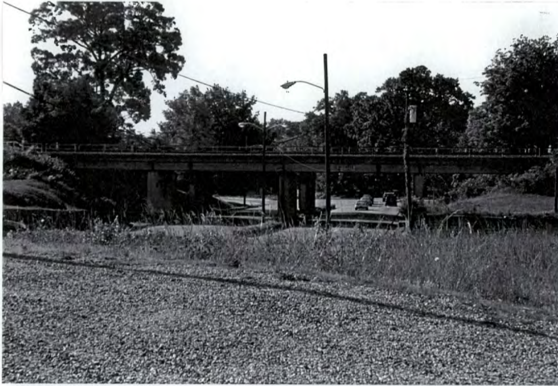
Plate 17: Railroad bridge over NC 127, south of downtown Hickory, looking north (outside of APE)
