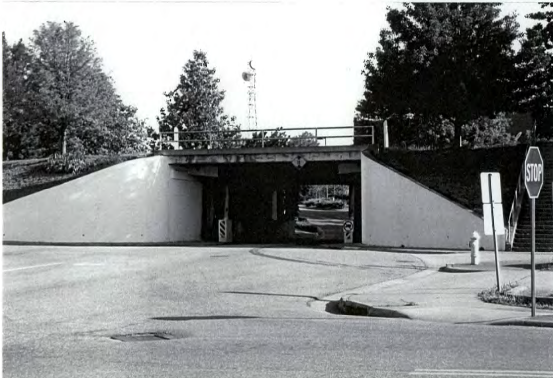
Plate 20: Railroad bridge over East 20th Street just west of NC 16, Newton, looking west (outside of APE)
