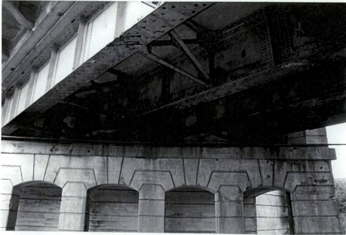
Plate 11: Highland Avenue Southern Railway Bridge – plate girders and east bent looking northwest
