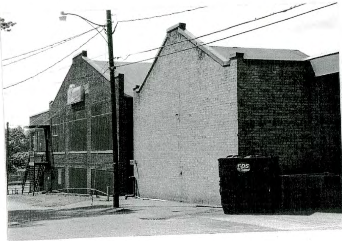
Plate 21: Whisnant Hosiery Mill – 1920s block at right, 1930s block at left, looking southwest
