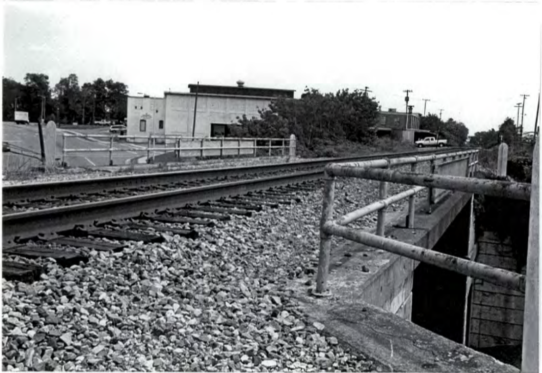
Plate 16: Highland Avenue Southern Railway Bridge – track and pipe railings looking northeast, Hickory Hosiery Mill in distance
