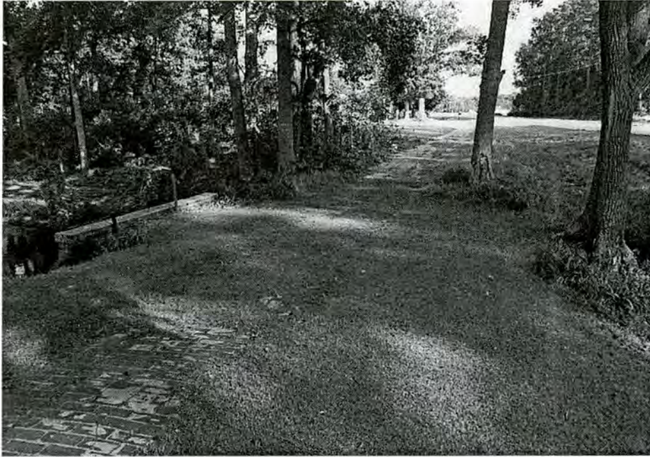
10. Brick Road (New Bern-Washington Brick Road Historic District). View S. Original brick culvert at L.
