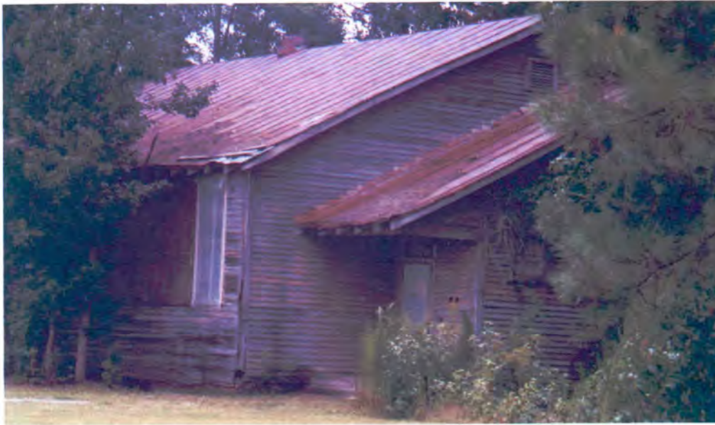
Figure 10. Property No. 213 – Jeffrey's School (NS 629). Part of south and east elevations. Photographed July 29, 2004.
