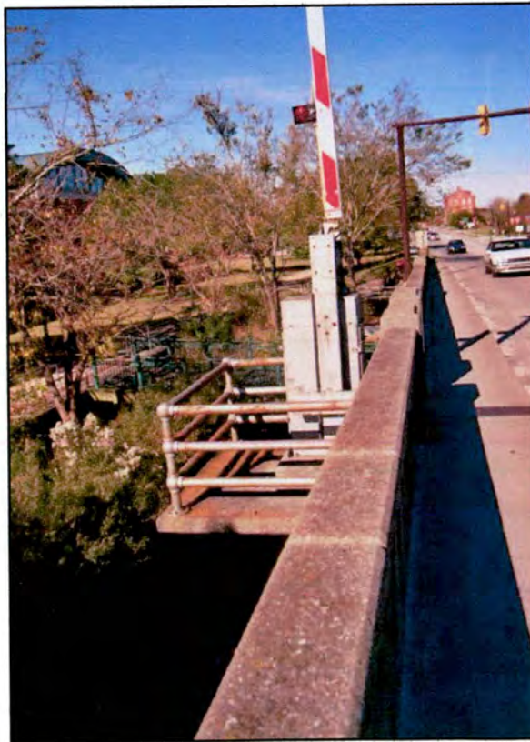
Figure 15: Traffic Barrier Platform, west side of bridge, looking north (convention center and Sparrow House in distance)
