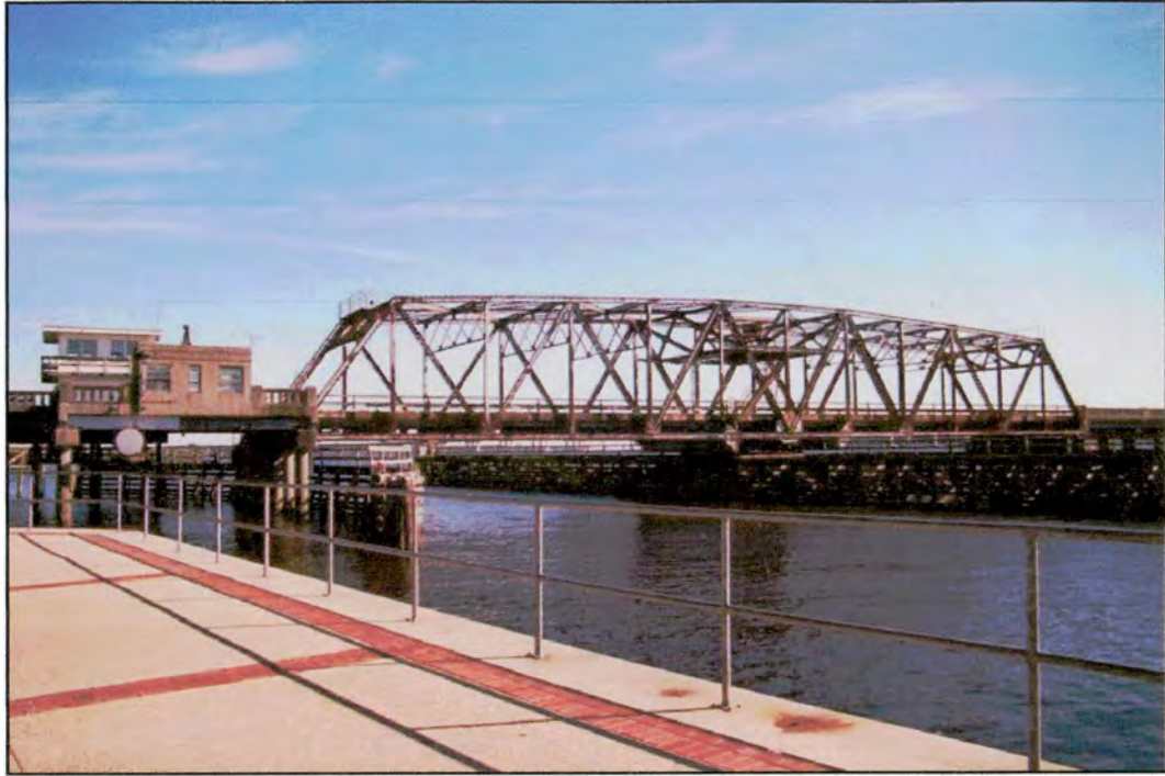
Figure 16: West elevation. Truss, moved operator's house, and 1955 bridge tender house (view from New Bern Convention Center promenade).
