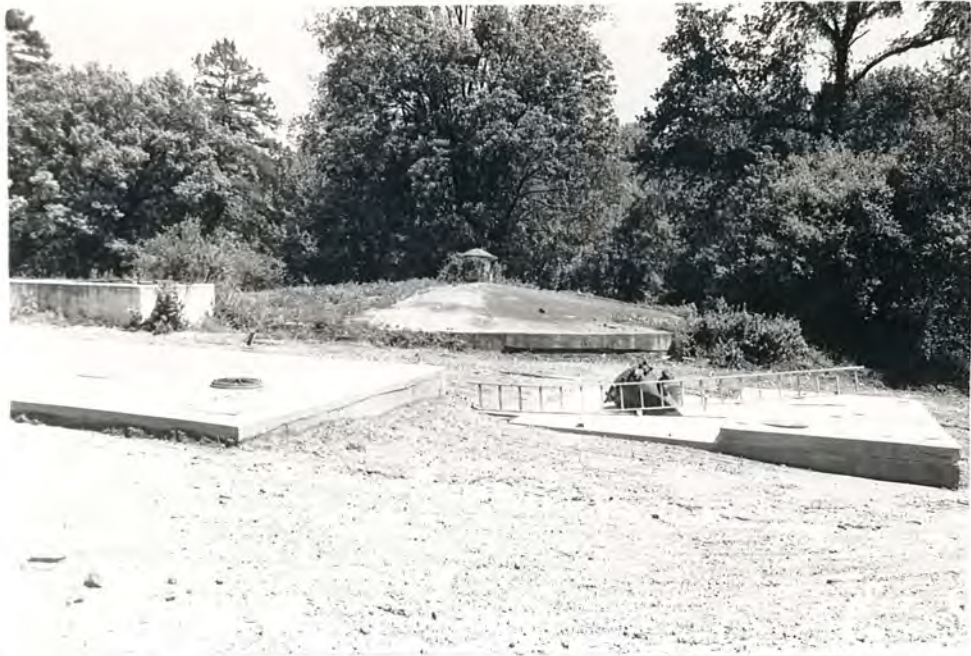
99. (C) High Point Waterworks, underground reservoir tank, view to S
