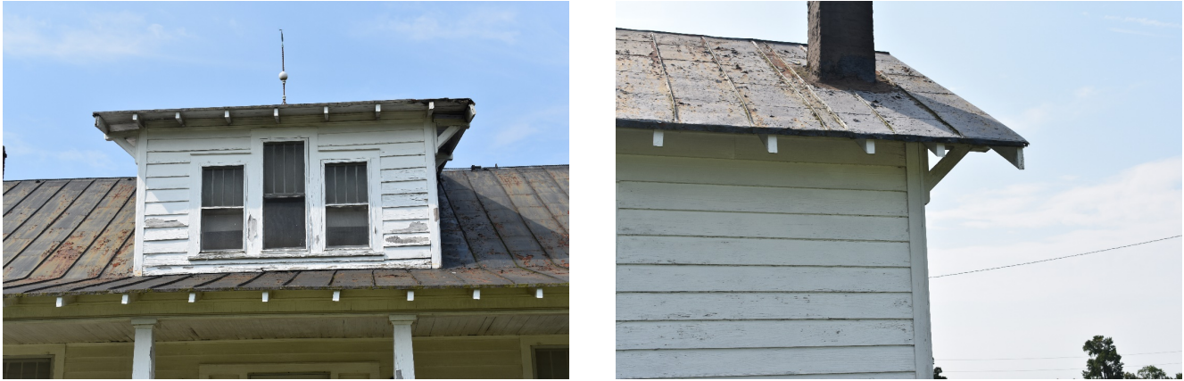
Figure 12: Left, detail of Raleigh Blowe Sr. House dormer, facing southwest; right, detail of weatherboard siding, cornerboard, and exposed rafter tails.
