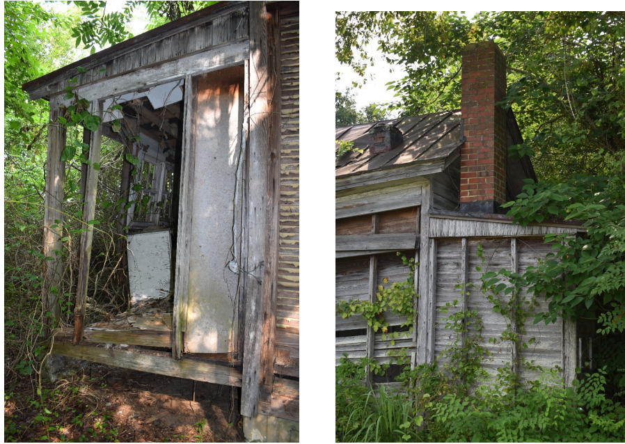
Figure 32: Left, looking northwest at secondary ell and southeast corner of the house; right, southwest corner of ell and secondary addition, facing southeast.
