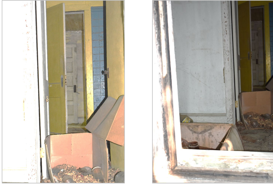
Figure 34: Left and right, interior views through secondary addition of the house, facing northwest.
