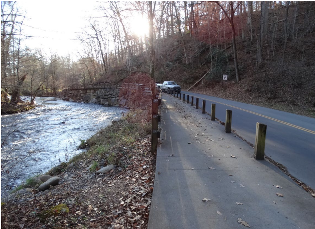
Figure 38: Stone retaining wall, fence, sidewalk, and guard posts at West Deep Creek Road, facing west (QE 2020).
