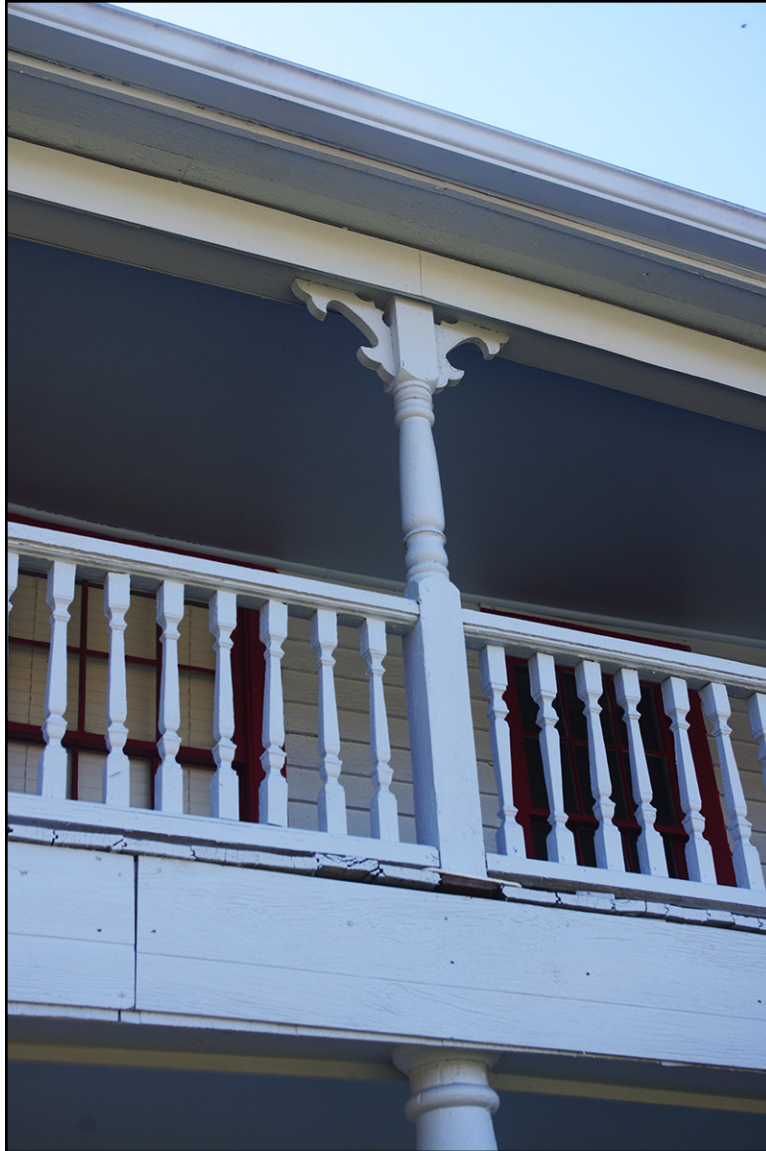
PLATE 13: Burch-Mathis House (YD0617), Detail of Decorative Bracket and Porch Posts, North Elevation, Yadkin County, North Carolina
