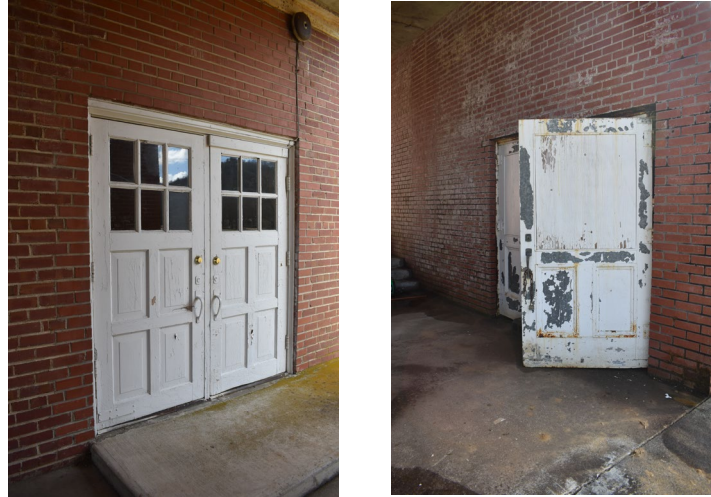
Figure 76: Left, original doors located underneath covered walkway leading into hallway of original building (viewpoint for interior hallway photos); right, doors located on north elevation of cafeteria addition, also situated underneath covered walkway (viewpoint for interior cafeteria photo).
