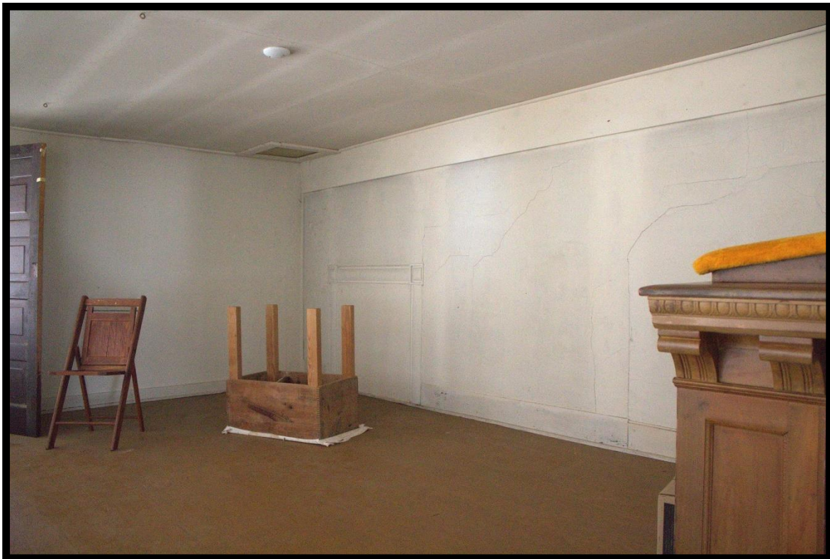
Figure 27: Union United Methodist Church, Interior, Enclosed Gallery, Looking Southwest. Note the Original Window Frame on the Right Wall near the Corner.
