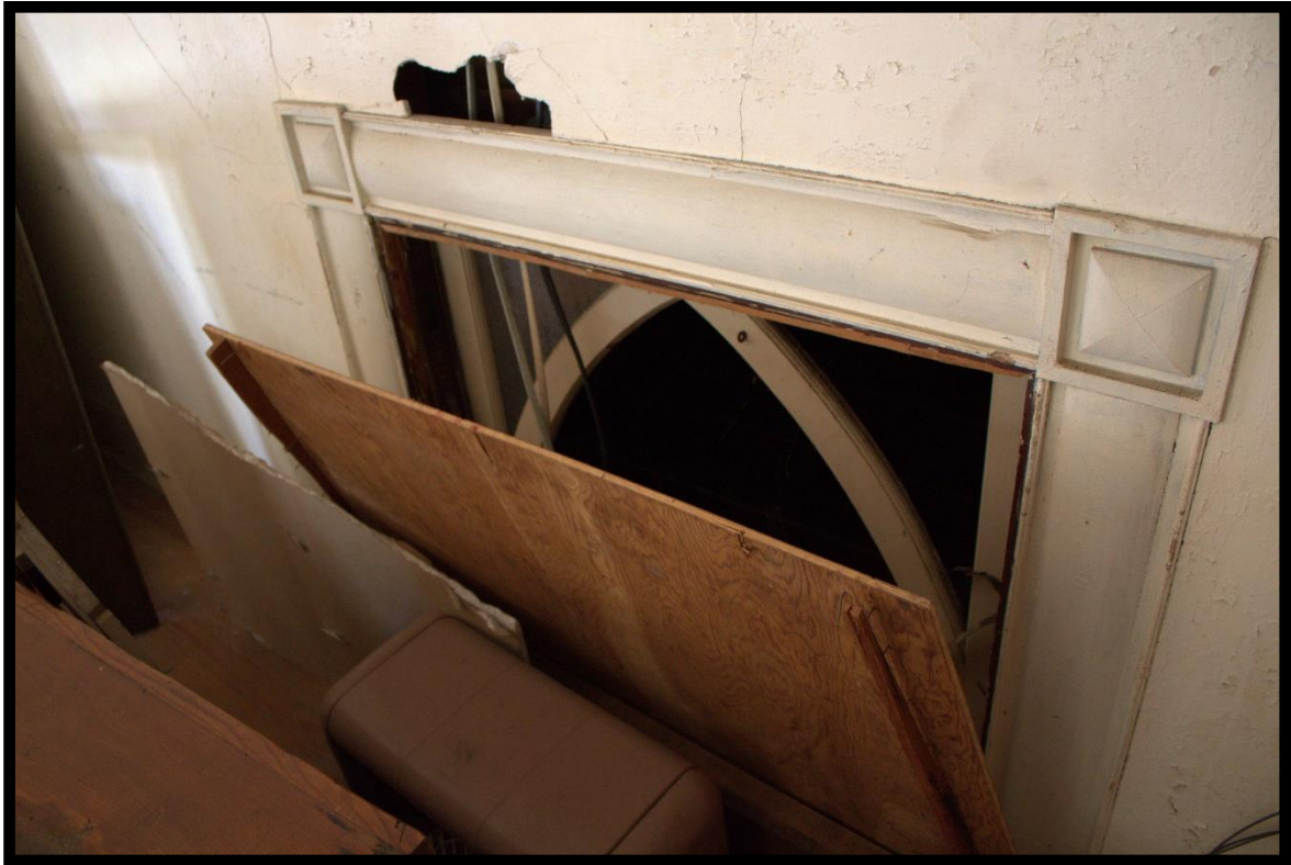
Figure 28: Union United Methodist Church, Interior, Enclosed Gallery, Detail of Original Window Sash.
