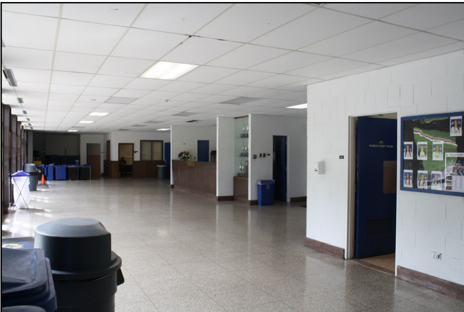
Plate 4.20 View of the lobby, concessions, and offices of the Chambers Gymnasium and Harrell Pool.
