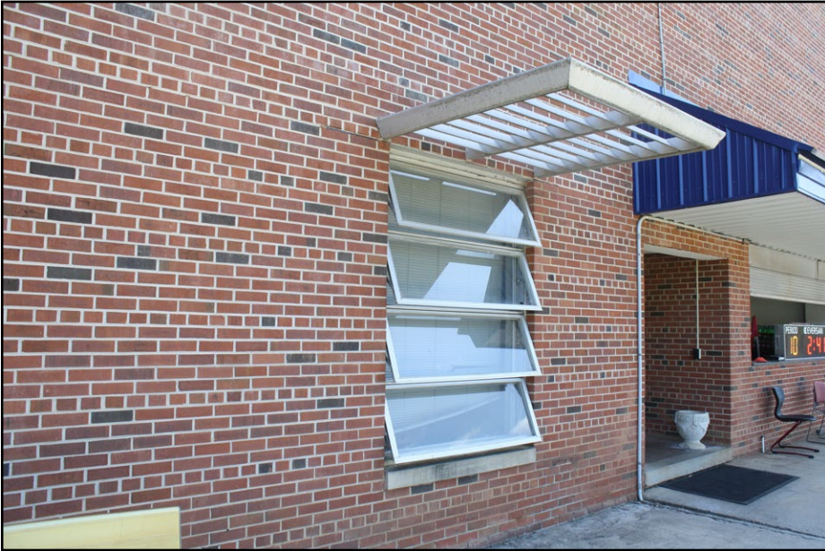
Plate 4.17 View of one rear entry door and window at the northwest corner of the Chambers Gymnasium and Harrell Pool.
