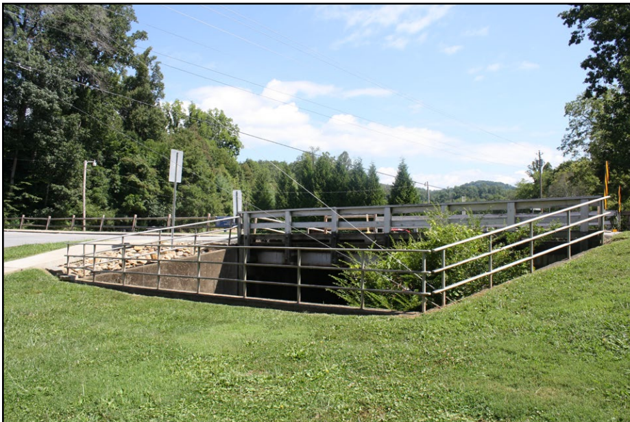
Plate 4.8 View of southwest side of Bridge No. 184 over Gabriel Creek at Bailey Street.
