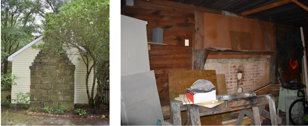
Figure 14. Left, view of kitchen chimney on eastern gable end; right, view into interior of building
