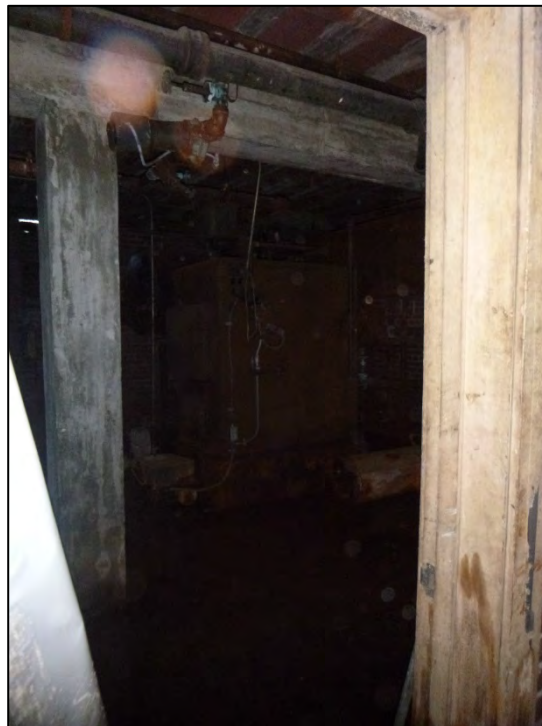
Figure 4.43. Mechanical equipment, facing northeast.
