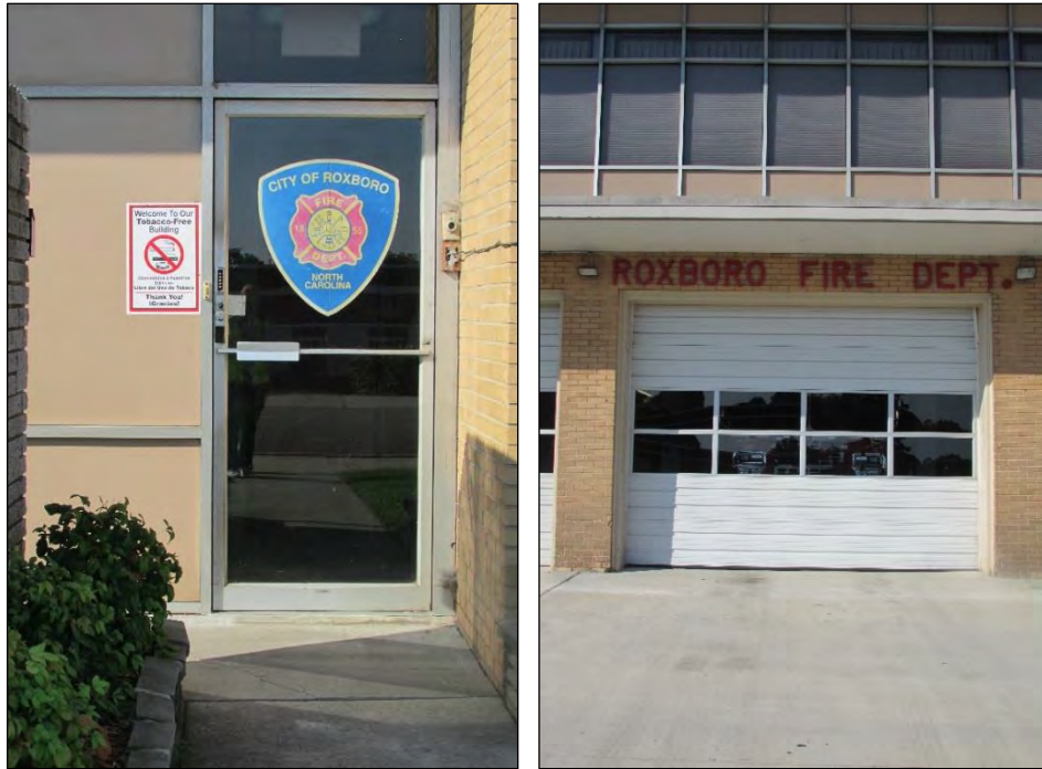
Photo 135: Fire Station Door (Left) and Garage Door (Right) Details on Northeast Elevation.
