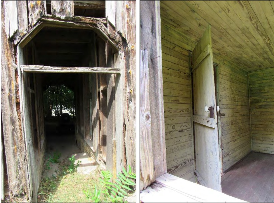
Photo 196: Entrance Detail on East Elevation (Left) and Door and Interior Detail of Northeast Room in Stable (Right).
