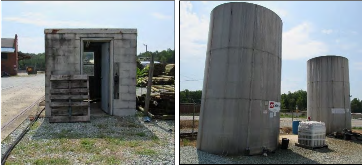
Photo 34: Weigh Station Structure, Facing West (Left). Concrete Storage Tanks Located Southeast of Building (Right).
