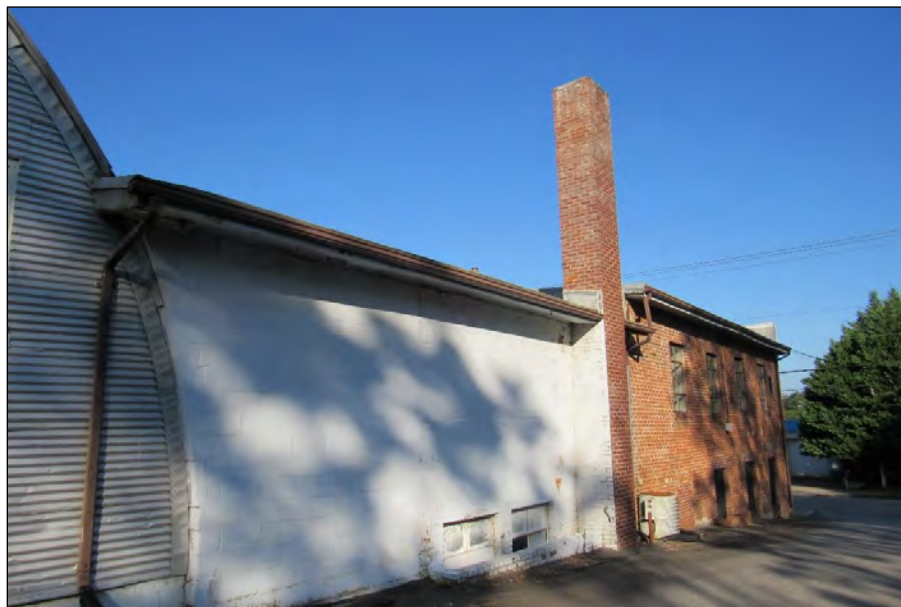
Photo 122: Detail of Building Addition and Quonset Hut Connection on the Northeast Elevation with Awning Window Left of Chimney Stack.
