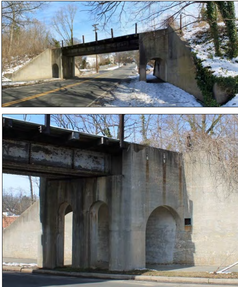
Photo 336: NS Railway Trinity Avenue Bridge, Looking East from W. Trinity Avenue (Top) and Pedestrian Walkway, Looking Northeast (Bottom). 759
