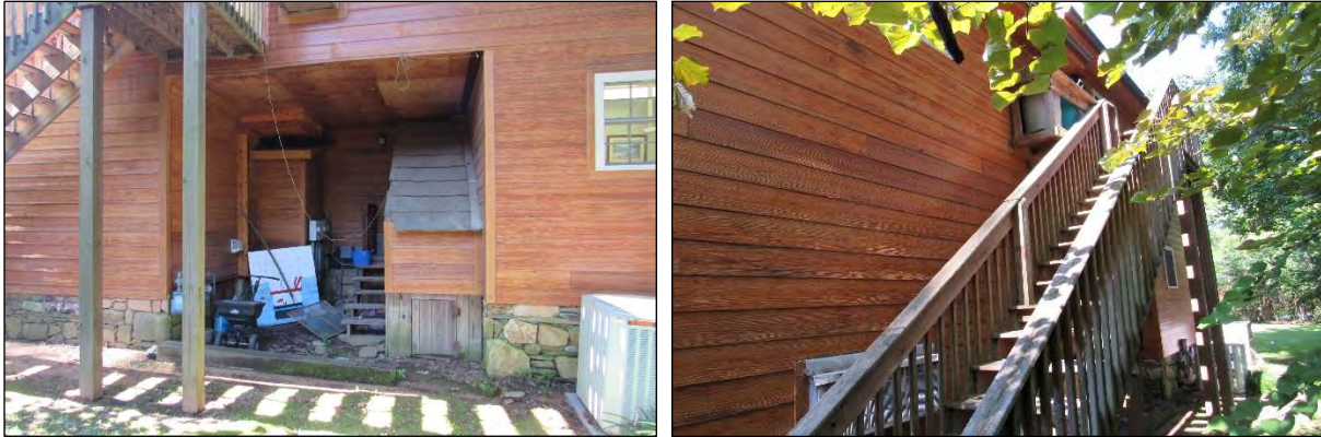
Photo 228: Recessed Area on Rear Elevation (Left) and Stairway on Rear Elevation to Second Floor (Right).
