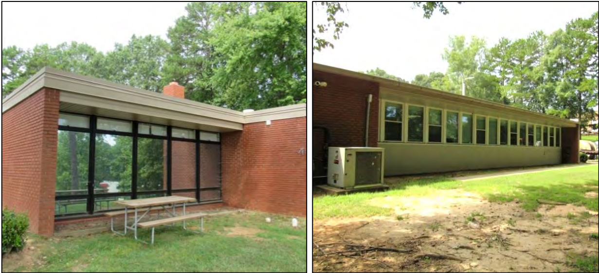
Photo 214: Original Windows on the East Elevation (Left) and Replacement Vinyl Windows on the North Elevation (Right).
