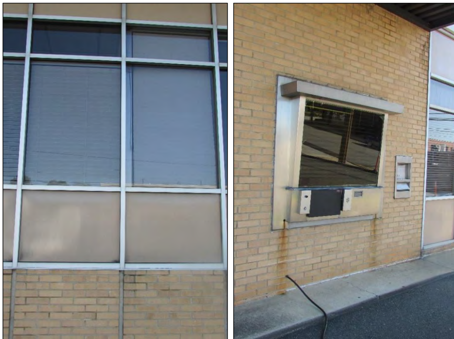
Photo 136: Window (Left) and Drive-Up Teller Window and Night Deposit Box (Right) Detail on Southwest Elevation.
