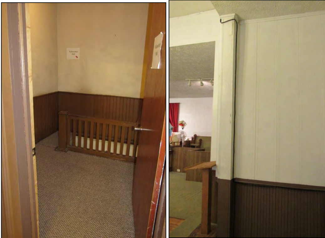
Photo 161: Access to the Staircase Looking Northeast (Left) and Surviving Pilaster and Wooden Paneling, Looking West (Right), Both within the Circa-1950 Addition.
