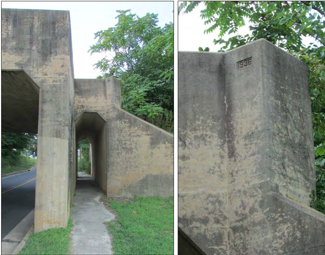
Photo 331: East Entrance to Pedestrian Walkway (Left) and Detail of Date Stamp, East Elevation (Right).
