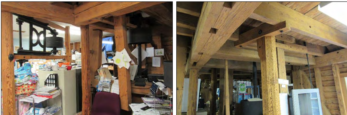
Photo 229: Interior Images of Dental Office Lounge and Mill Machinery.
