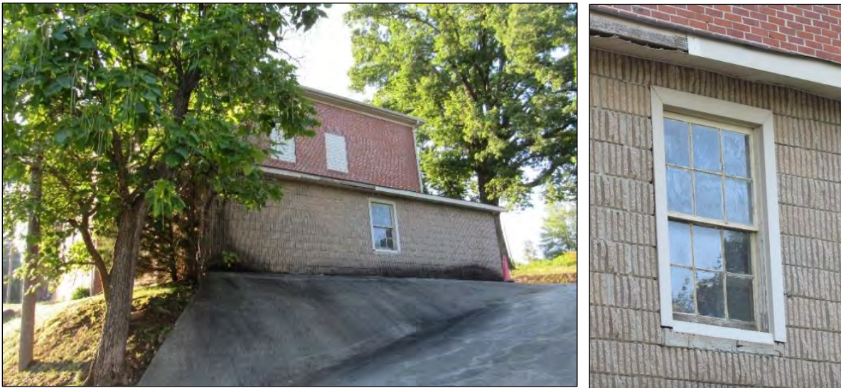
Photo 312: View of Rear Addition, Looking East (Left) and Detail of Window (Right).
