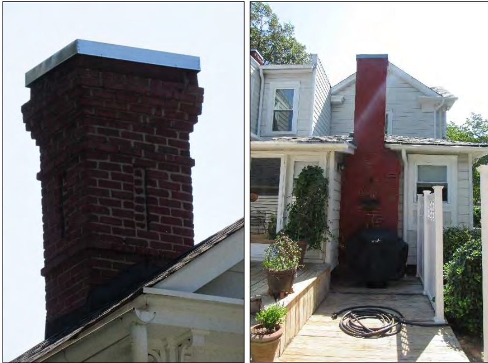
Photo 248: Corbeled Chimney Detail, Looking East (Left) and Stepped Base Chimney Detail, Looking East (Right).
