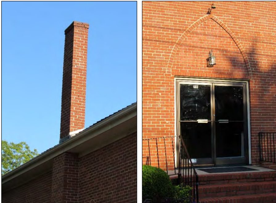
Photo 308: Chimney Detail, Looking West (Left) and Primary Entrance Detail, Looking West (Right).
