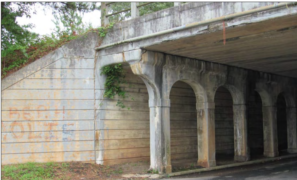
Photo 338: Atlantic Coast Line Railroad Underpass on Former Raleigh & Gaston Rail Corridor (NC0008) at U.S. Highway 158/401 S near Norlina, North Carolina.
