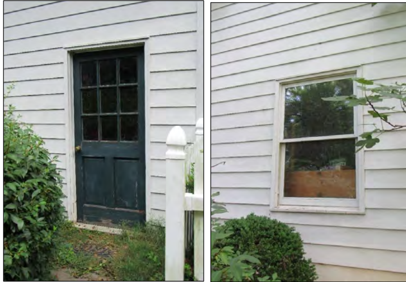
Photo 198: Door Detail on South Elevation (Left) and Window Detail on West Elevation (Right) of Circa-1980 Garage.
