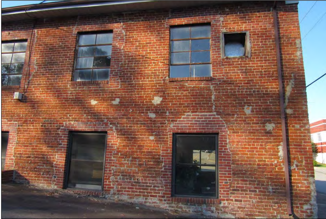
Photo 120: Detail of Fenestration on Northeast Elevation. Note the modifications to the exterior windows sizes, indicated by the patchwork of brick repairs.
