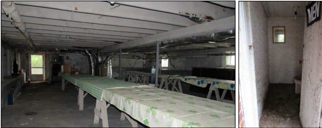
Photo 97: View of Basement, Looking North (Left), and View of Bathroom, Looking Southeast (Right).
