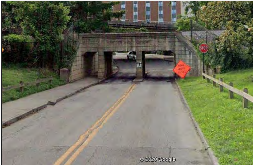
Photo 335: View Looking East at Circa-1938 N&W Railway Underpass Over Wiley Drive SW in Roanoke, Virginia. 750
