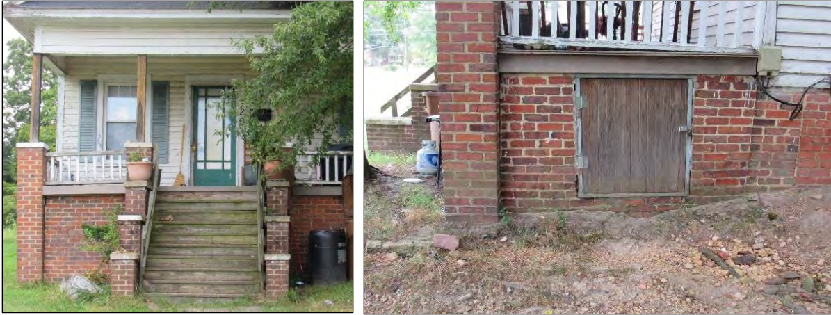
Photo 298: Entrance Detail on West Elevation (Left) and Foundation Detail on South Elevation (Right).
