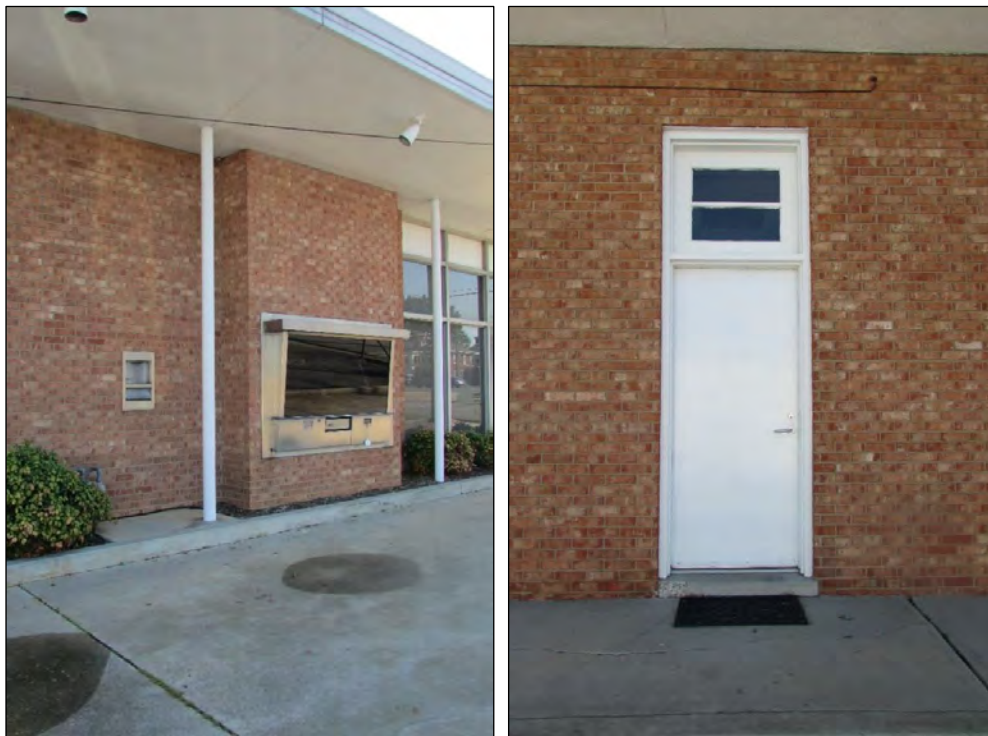
Photo 175: Night Deposit and Teller Window on the Southwest Elevation (Left) and Rear Entrance Door and Transom (Right) on the Northeast Elevation.
