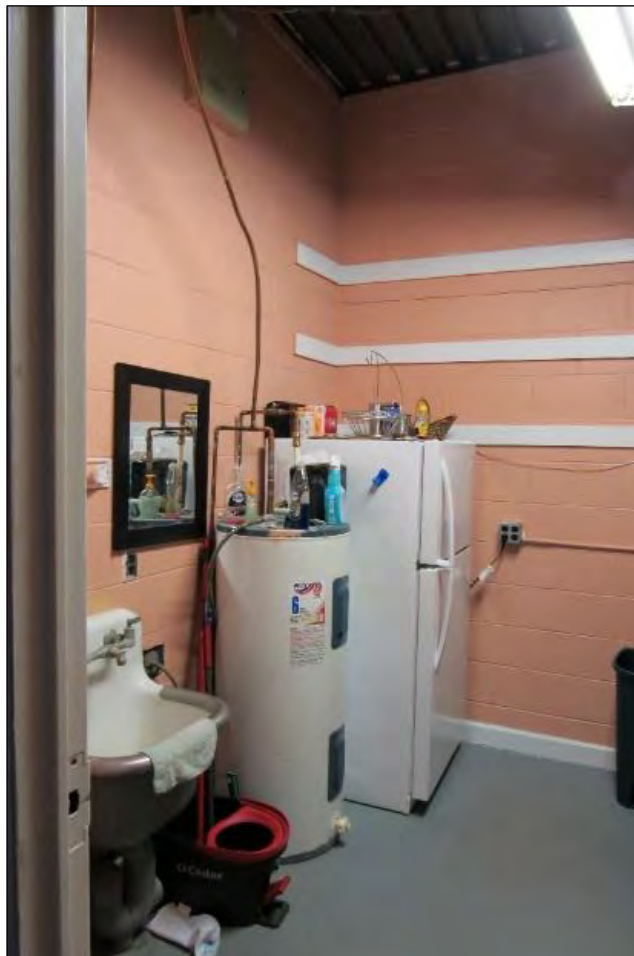
Photo 42: View of Office Space, Facing Southeast (Top), and Storage Room Facing South (Bottom).
