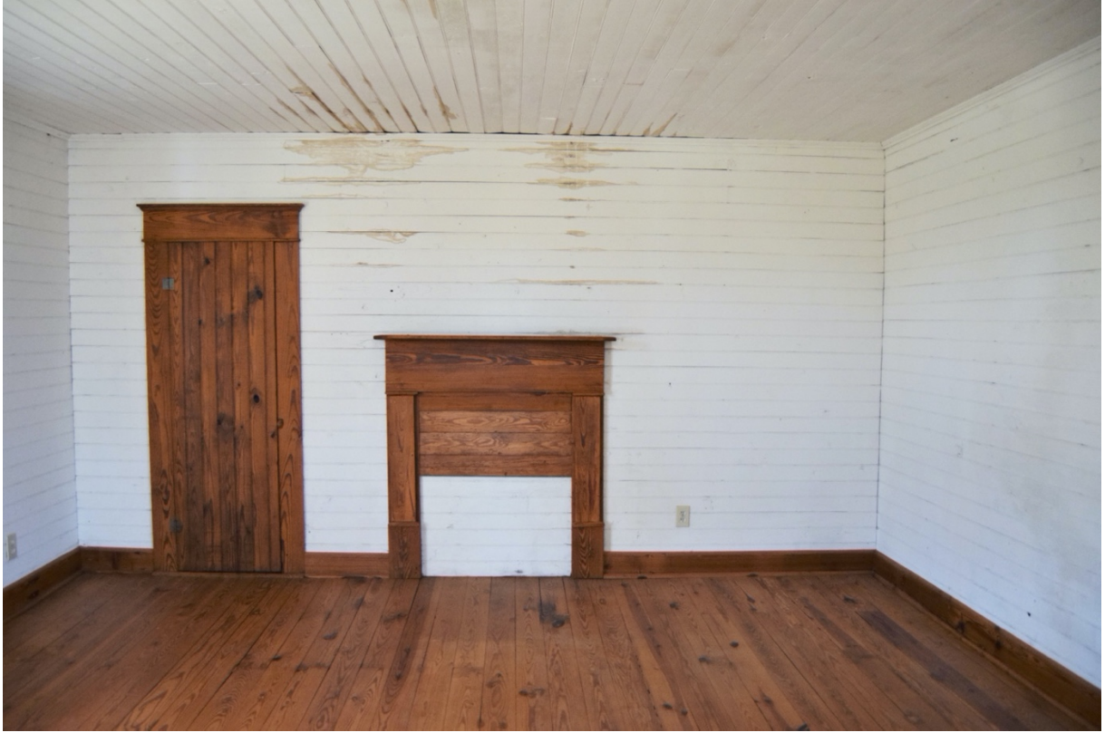
Dwelling, Bartley Yates Farm, front west room at second floor, view to south.
