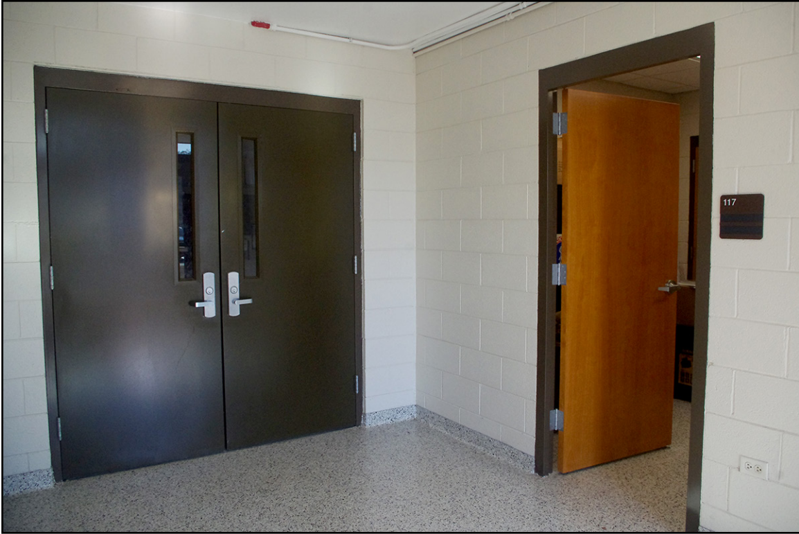
PLATE 53: Interior of Entry Leading to Drill Hall, Facing North, Nashville National Guard Armory (NS1563), Nash County, North Carolina
