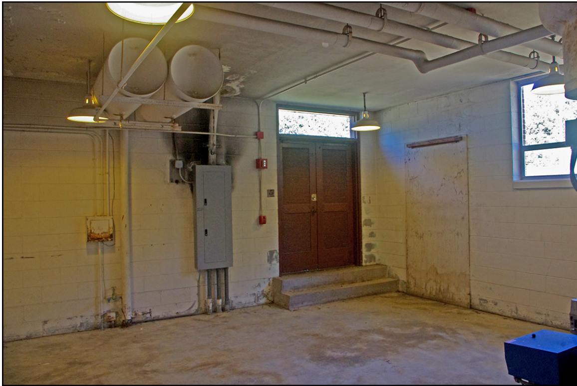
PLATE 71: Interior of Boiler Room, Facing Northwest, Roseboro, National Guard Armory (SP0769), Sampson County, North Carolina
