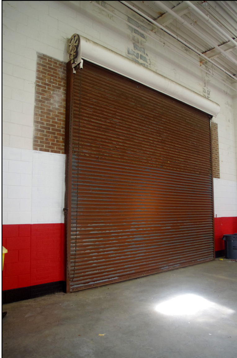
PLATE 70: Detail of Original Metal Roll-up Garage Door in Drill Hall, Facing Northwest, Roseboro National Guard Armory (SP0769), Sampson County, North Carolina
