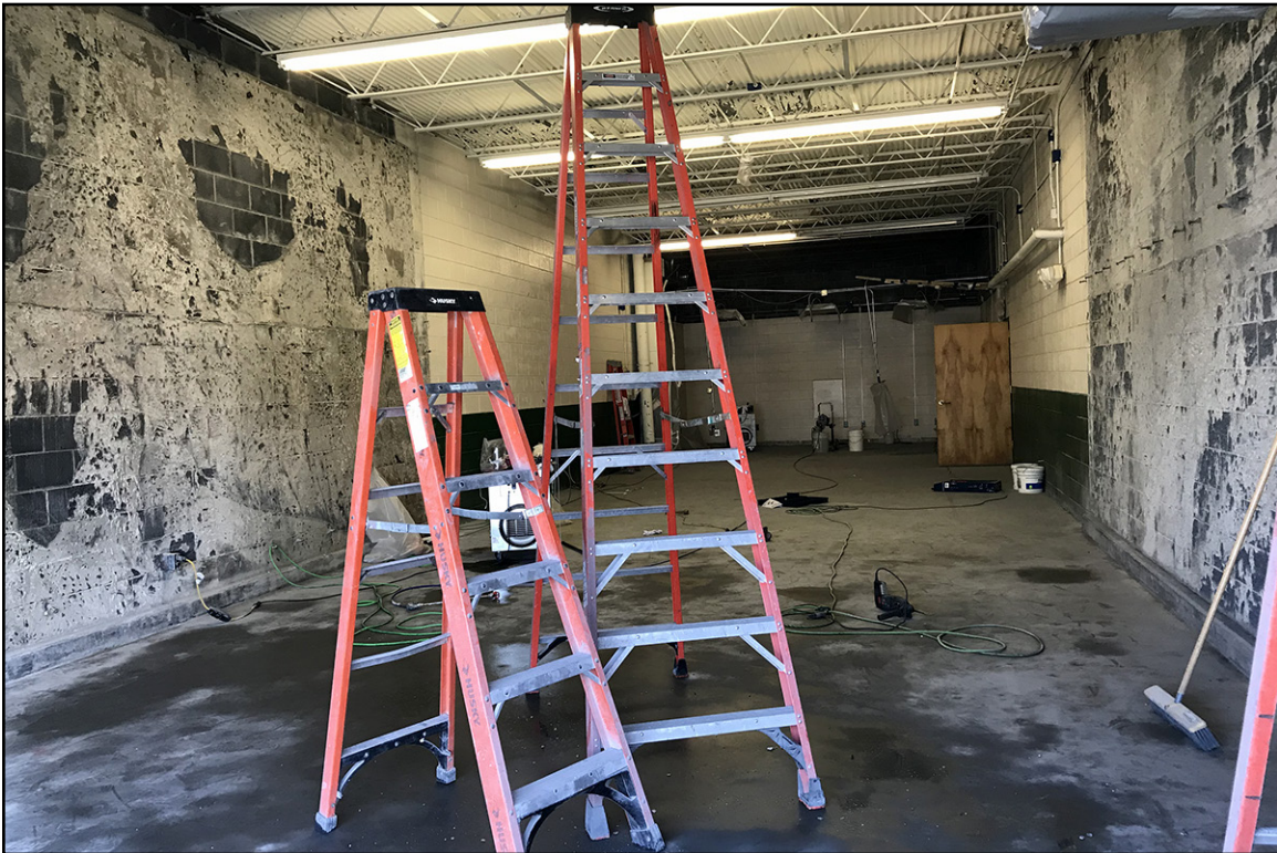
PLATE 33: Interior of Former Rifle Range, Facing East, Greenville National Guard Army (PT3357), Pitt County, North Carolina
