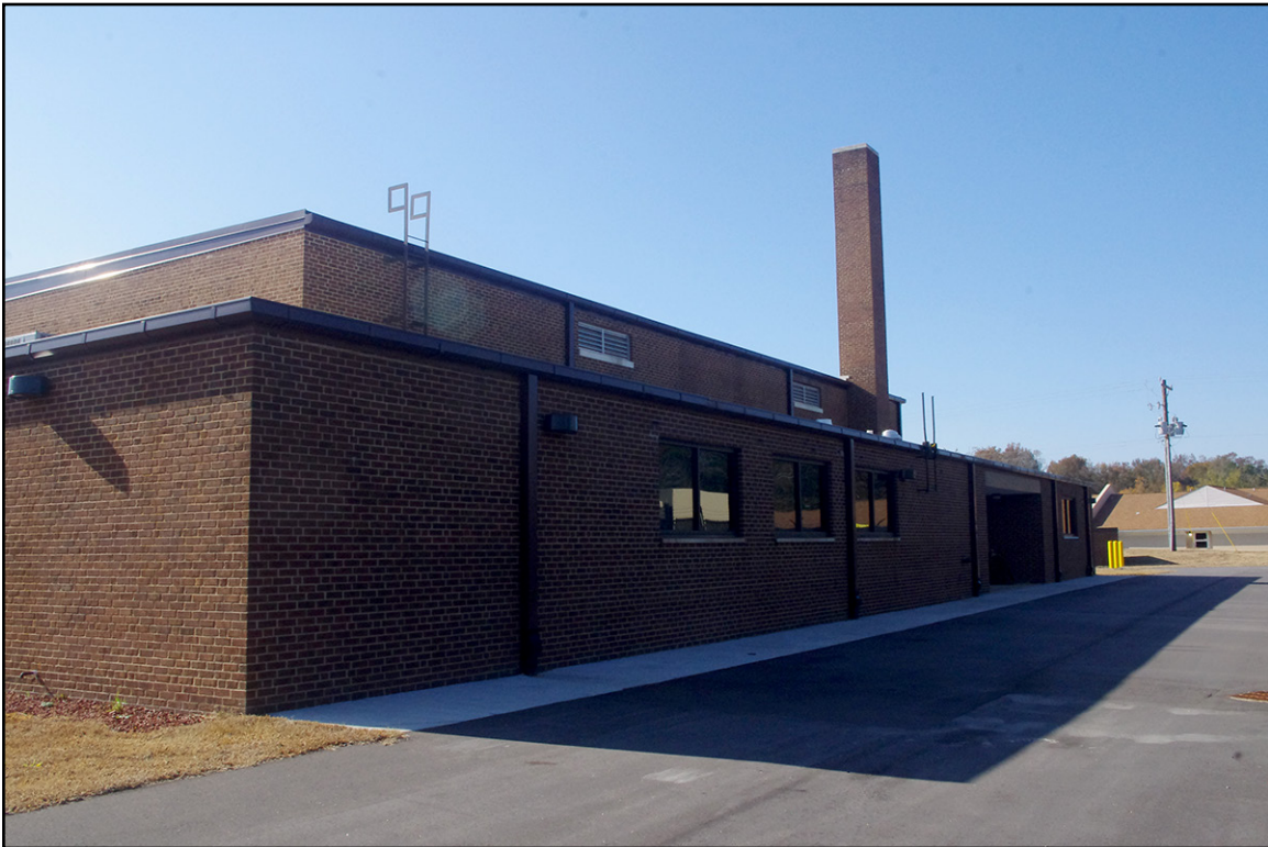
PLATE 50: North Elevation, Oblique View, Nashville National Guard Armory (NS1563), Nash County, North Carolina
