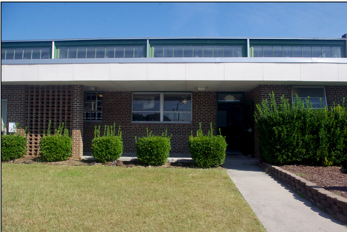
PLATE 29: Detail of Recessed Portion of South Elevation, Greenville National Guard Armory (PT3357), Pitt County, North Carolina
