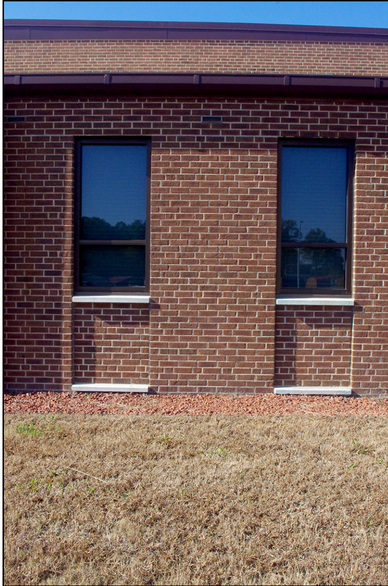
PLATE 47: Window Detail of East Elevation, Nashville National Guard Armory (NS1563), Nash County, North Carolina
