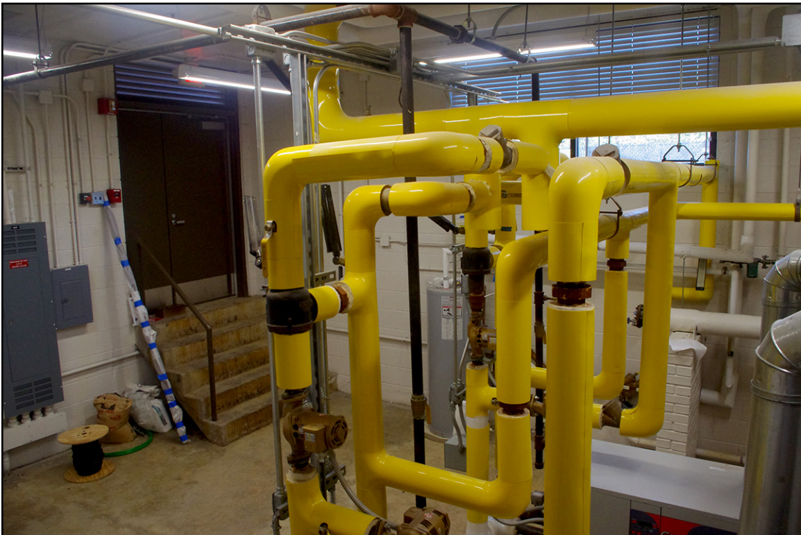
PLATE 56: Interior of Boiler room, Facing Northwest, Nashville National Guard Armory (NS1563), Nash County, North Carolina
