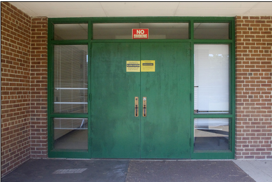
PLATE 27: Entrance Detail, East Elevation, Greenville National Guard Armory (PT3357), Pitt County, North Carolina
