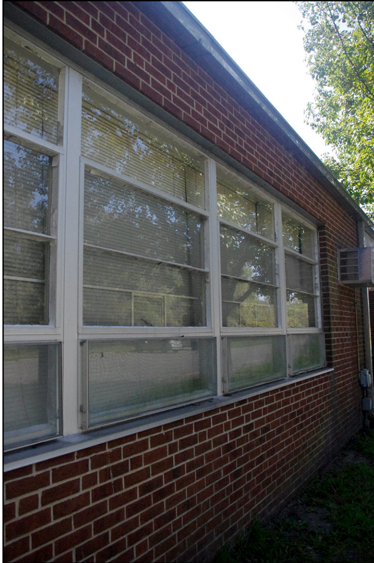
PLATE 16: Detail of Window Block, West Elevation, Fremont National Guard Armory (WY1458), Wayne County, North Carolina
