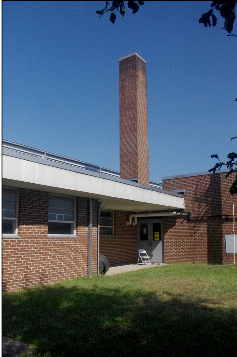
PLATE 20: Detail of Recessed Portion of East Elevation, Fremont National Guard Armory (WY1458), Wayne County, North Carolina
