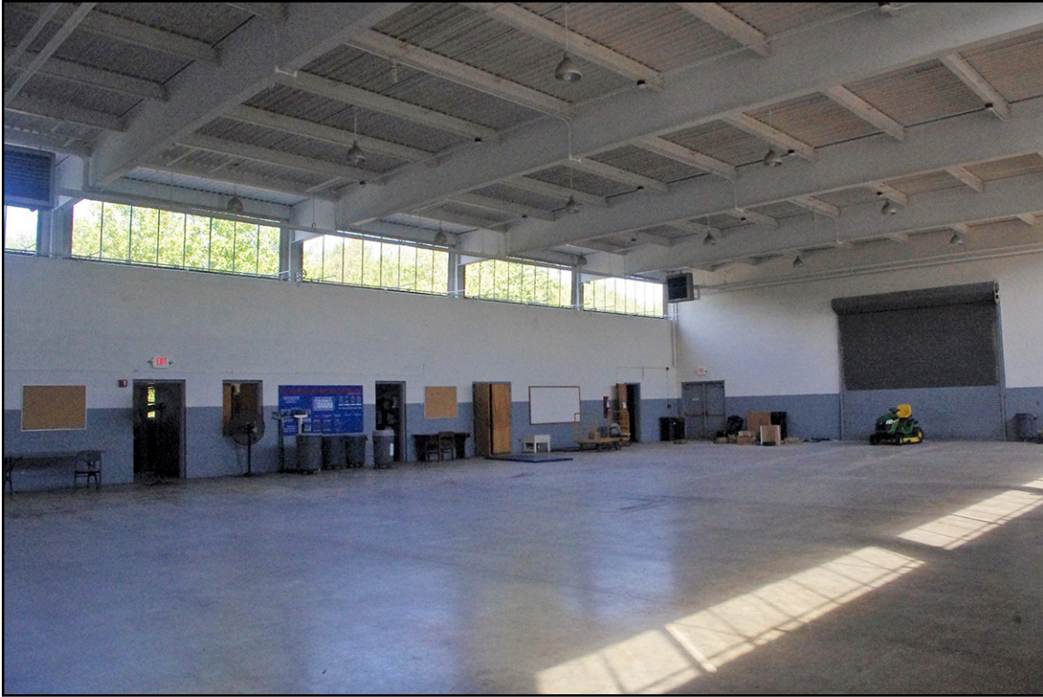
PLATE 21: Interior of Drill Hall, Facing Northwest, Fremont National Guard Armory (WY1458), Wayne County, North Carolina
