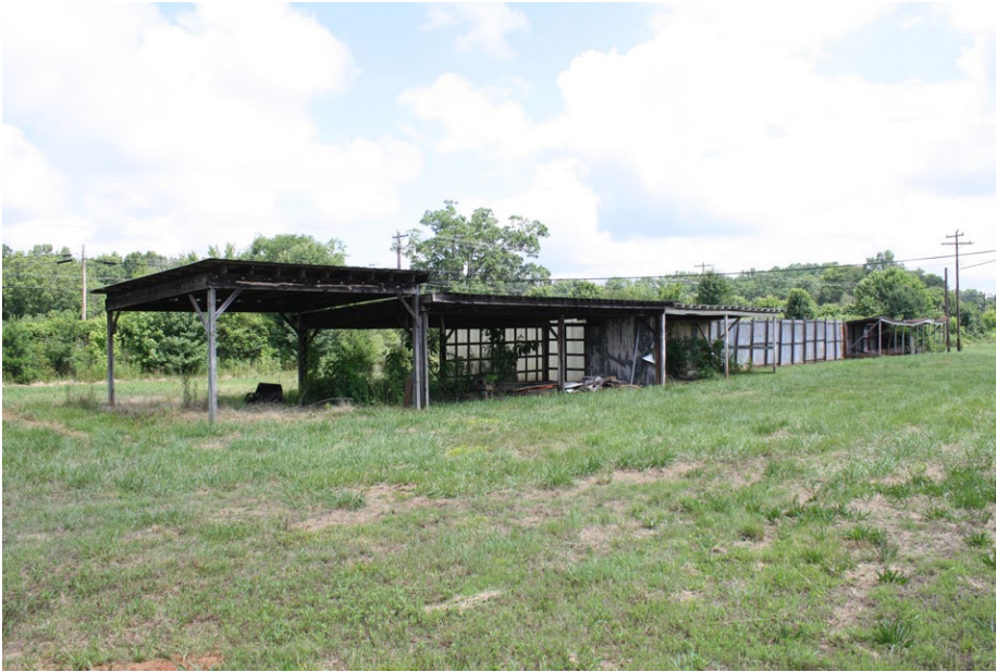
Plate 4.43: View of the storage sheds along the northwest edge of the parcel boundary.
