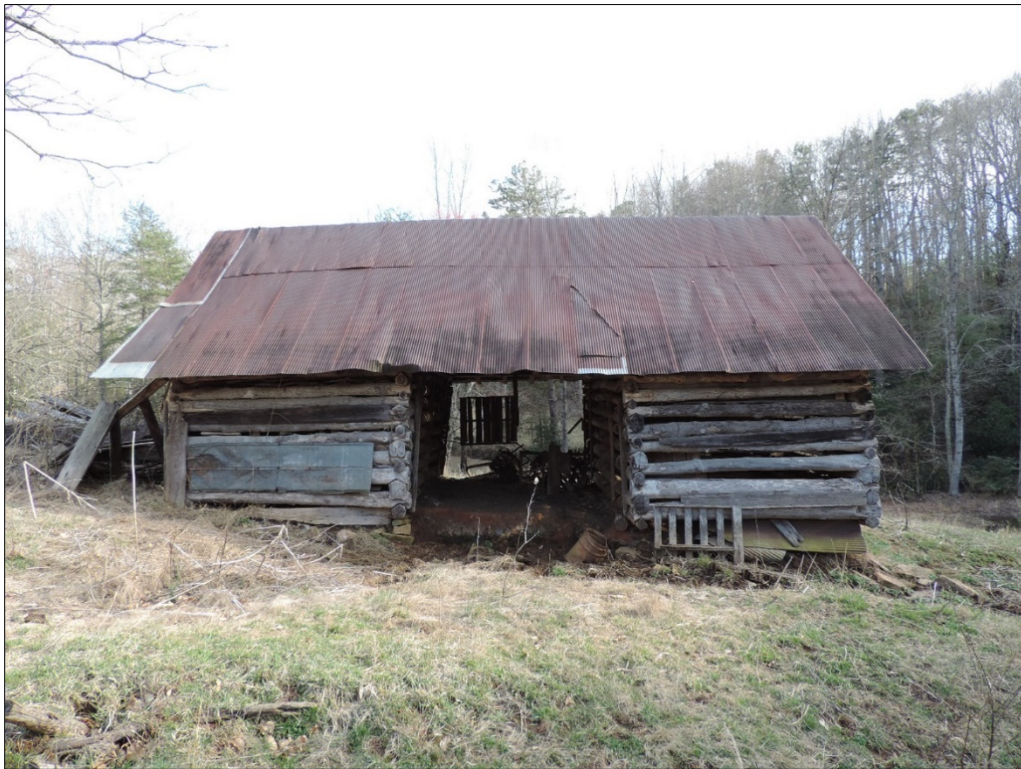
Figure 40: Northern elevation of nineteenth century double-pen log barn, twentieth century standing seam metal roof
