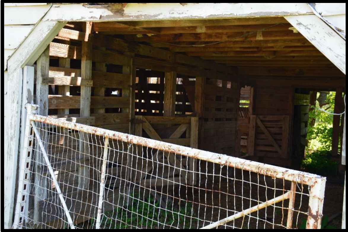
Figure 15: Ellis Tenant House, Barn, Interior of Ground Floor Showing Animal Pens Along the Side of the Alleyway.
