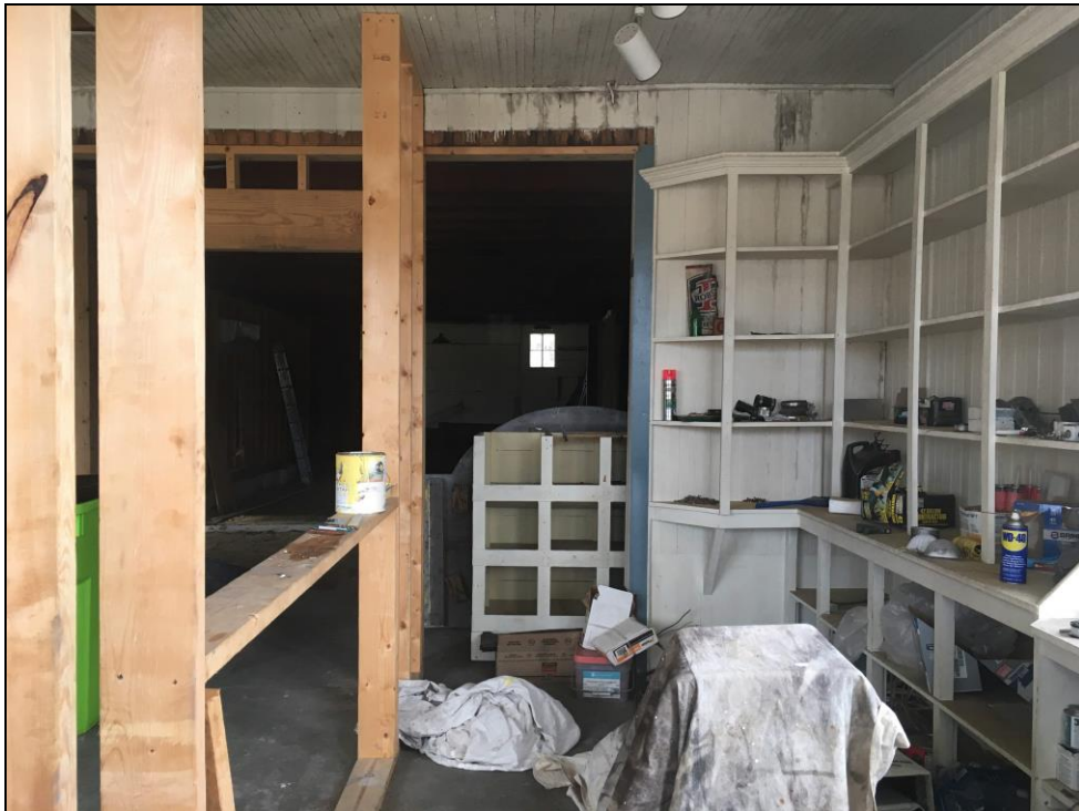
Figure 16: Interior, detail of original shelving on the north wall of the one-story restaurant addition, looking west.
