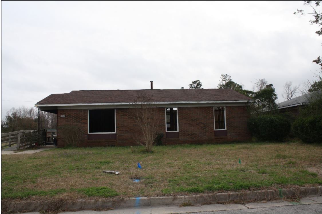
Figure 26: 2606 Robeson Street (House #14) side-gable, side entrance model, derelict
