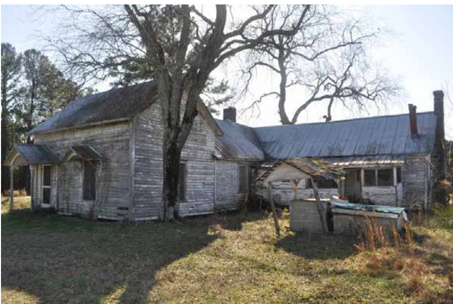
Plate 5.3: View of the rear, including side addition, main block and ell of the Maynard Farm house.
