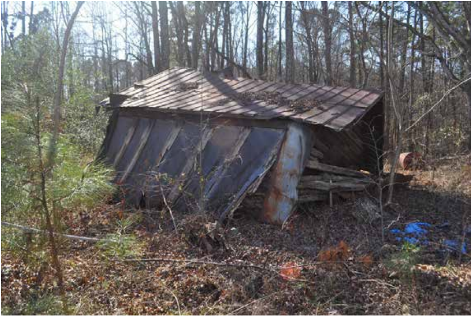
Plate 5.19: View of a deteriorating log barn on the subject parcel.
