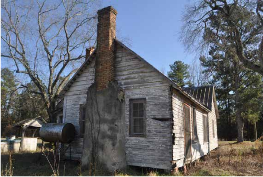
Plate 5.4: View of the rear ell (northwest and southwest sides) of the Maynard Farm house.
