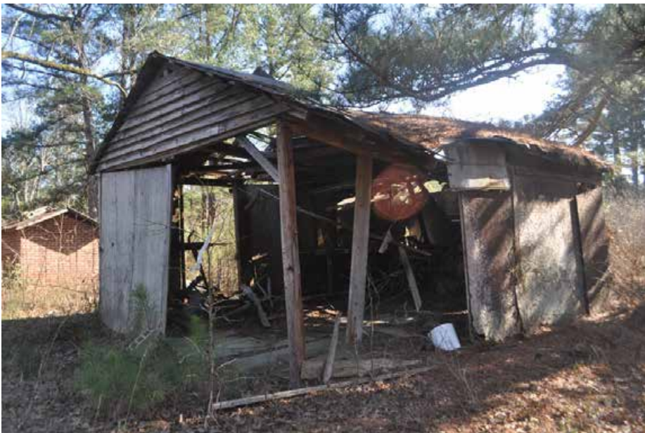
Plate 7.10: View of a deteriorating shed on subject parcel.
