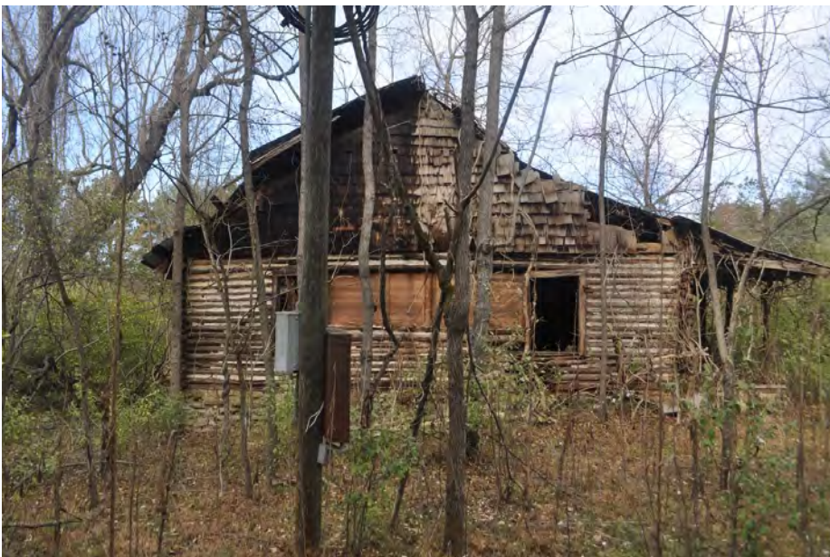
Plate 6.5: South side of Log House. Photo view: North Photographer: Ellen Turco Date: November 20, 2019
