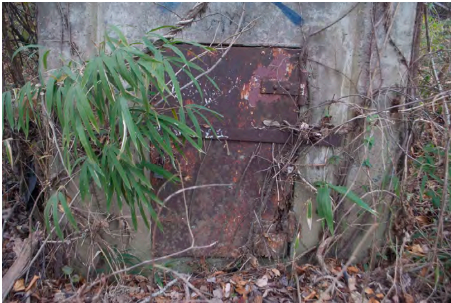
Plate 4.4: Door at the base of the east side of the French Broad River Gaging Station.
