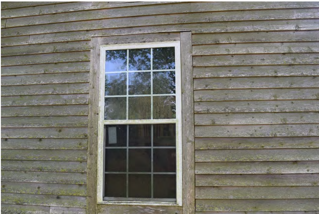
James S. and Sarah R. Heritage House, Rear (East) Elevation, Replacement Window and Siding, Looking West.
