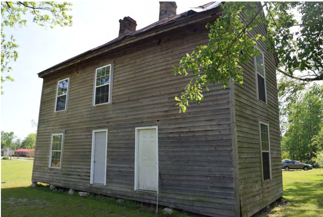
James S. and Sarah R. Heritage House, Rear (East) Elevation, Looking West.
