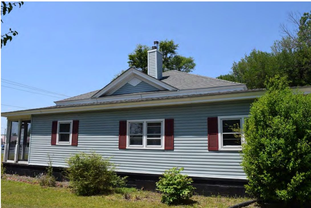
Jefferson D. Greer House, Side (South) Elevation, Showing Enclosed Wraparound Porch, Looking North.
