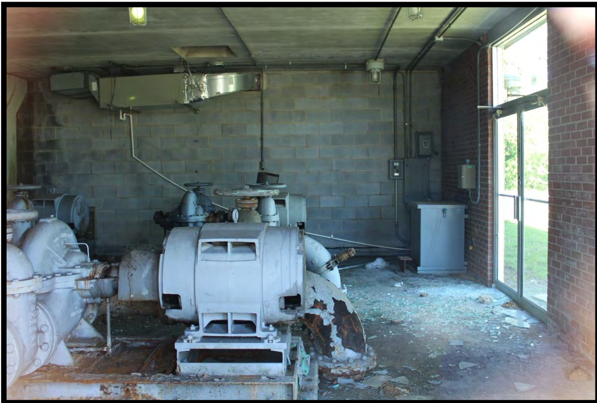
Figure 36: Lumberton Water Treatment Plant, Mechanical Building, Interior. Note concrete block dividing wall.
