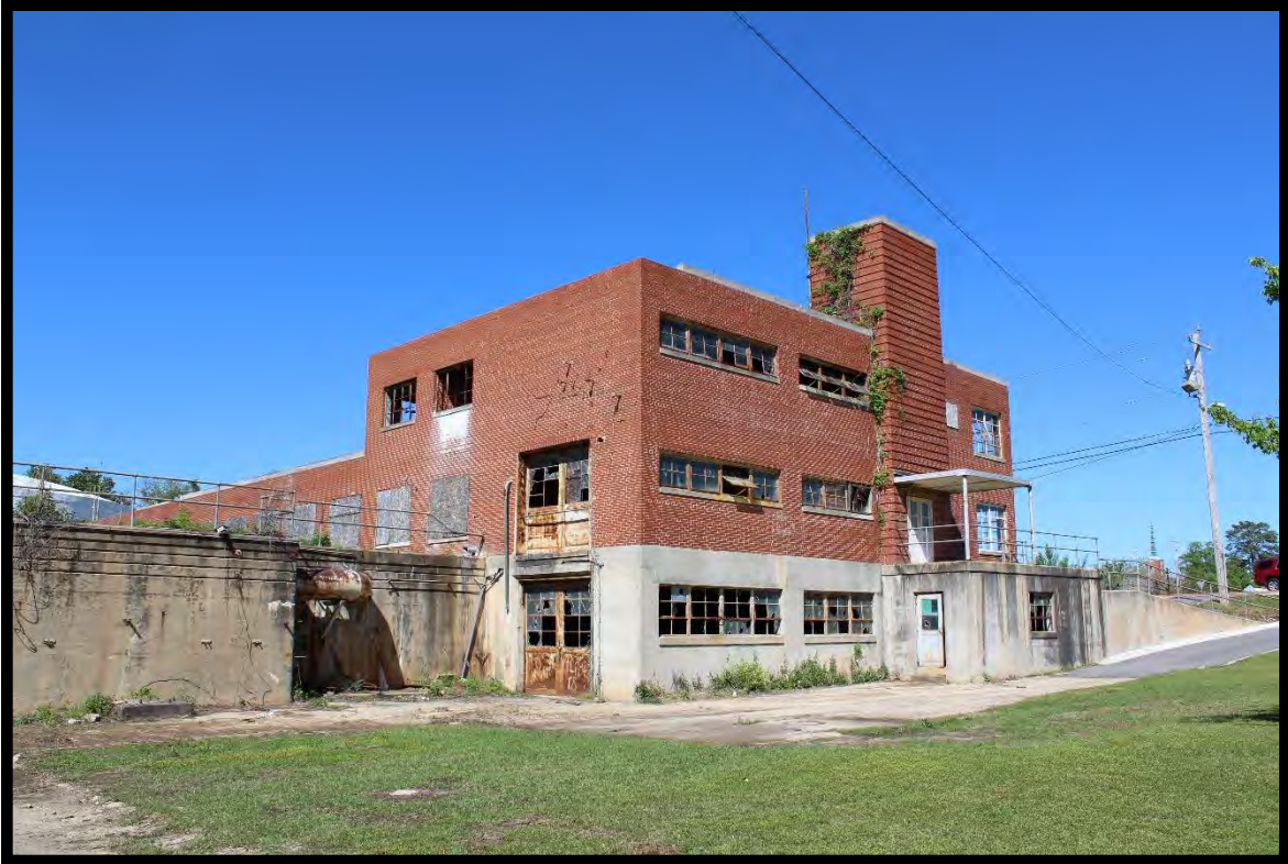
Figure 25: Lumberton Water Treatment Plant, Looking Northeast.
