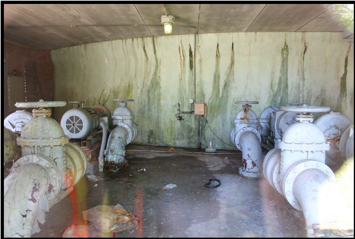
Figure 35: Lumberton Water Treatment Plant, Mechanical Building, Interior. Note curved wall of water tank.
