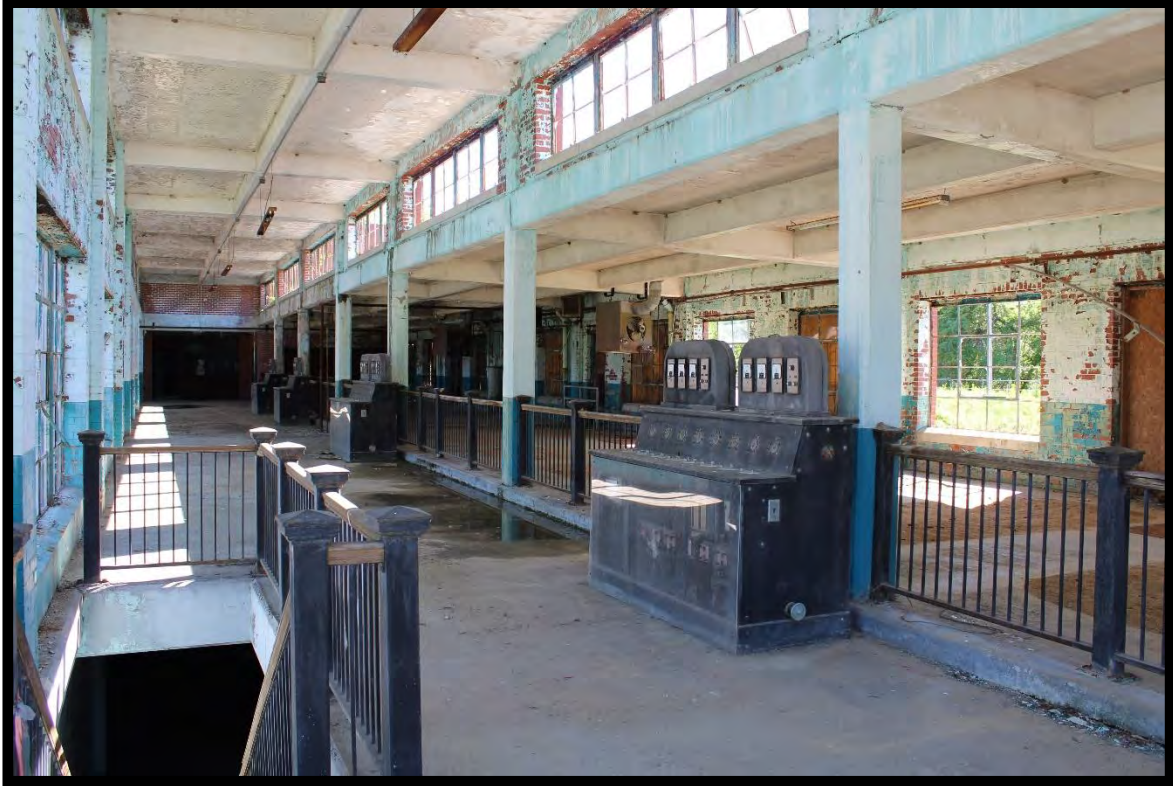
Figure 31: Lumberton Water Treatment Plant, Interior, Control Cabinets.
