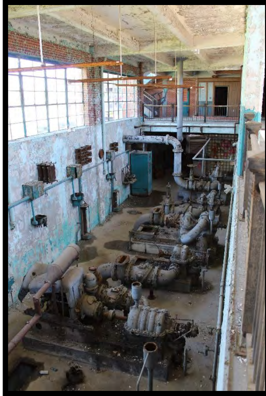
Figure 29: Lumberton Water Treatment Plant, Interior, Mechanical Equipment.
