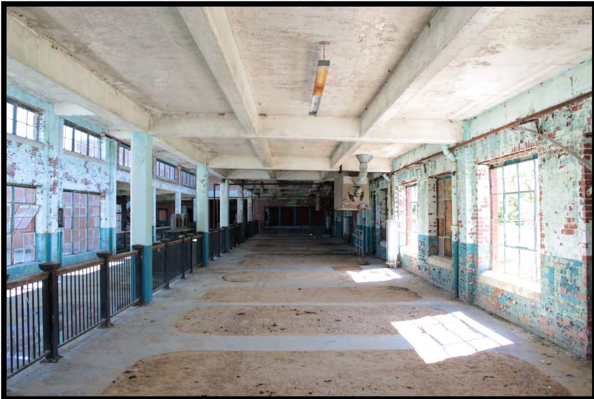
Figure 30: Lumberton Water Treatment Plant, Interior, Filled Water Basins.
