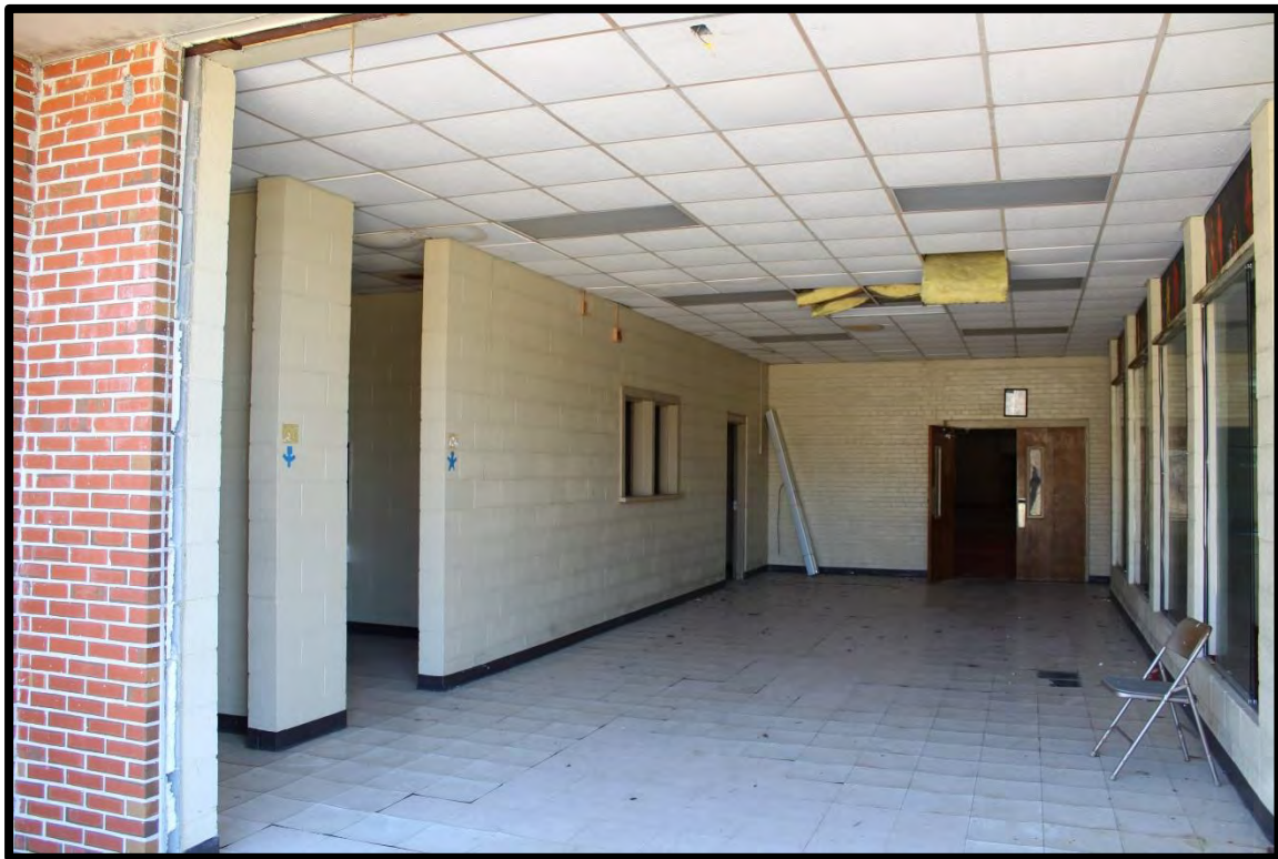
Figure 81: Tabor City School, Gymnasium, Rear Addition Added to Provide a Handicap-Accessible Entrance and Restrooms.
