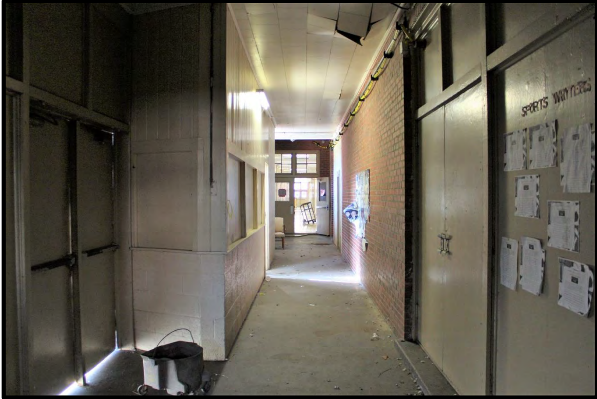
Figure 80: Tabor City School, Hyphen Between Gymnasium and 1948 High School Showing Interior and Exterior Entry Doors and Concession Stand.
