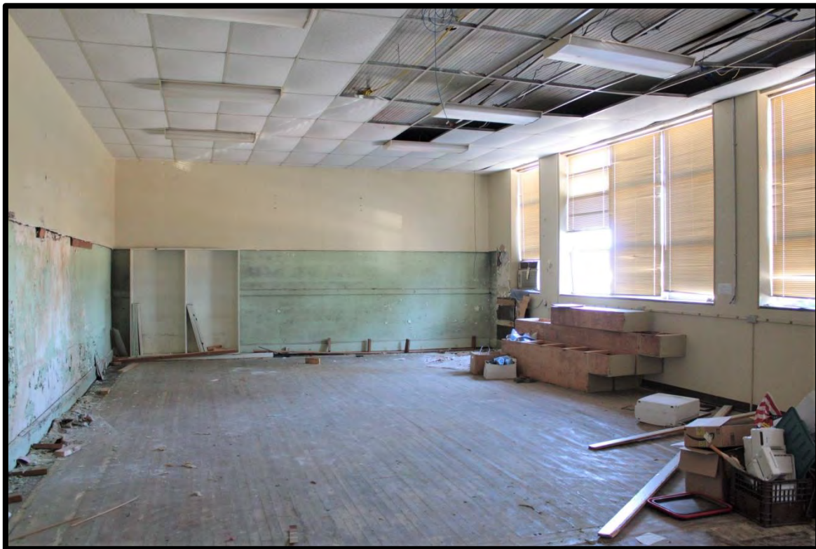
Figure 16: Cerro Gordo School, Classroom with Original Wooden Flooring, Plaster Walls, and Wooden Beadboard Ceiling Exposed.
