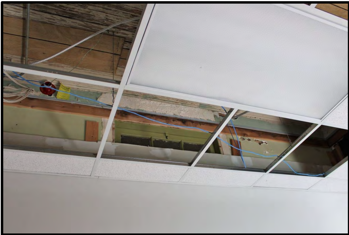
Figure 64: Tabor City School, Original Beadboard Ceiling, Wooden Trim, and Transom Concealed by Modern Materials.
