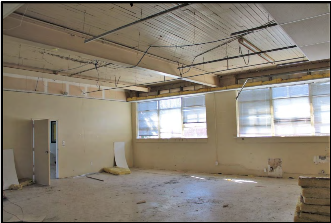
Figure 88: Tabor City School, Occupational Trades Building, Original Portion of Building Showing Exposed Original Material.
