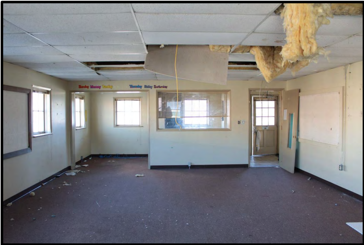
Figure 20: Cerro Gordo School, Agricultural Building, Classroom, Small Front Room and Entry Bay.
