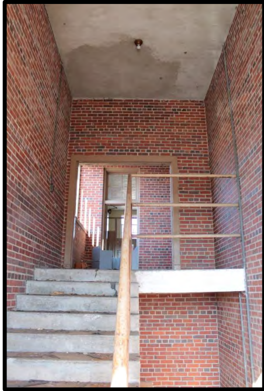
Figure 75: Tabor City School, 1948 High School, West Stairwell. Note Entrance to Restroom in Background.
