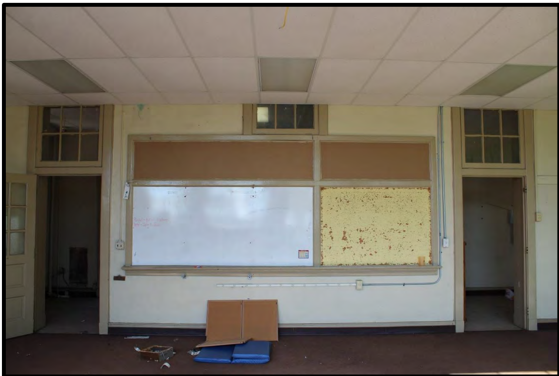
Figure 72: Tabor City School, 1948 High School, Original Layout with Two Entry Doors, a Transom, and a Built-In Lesson Board.
