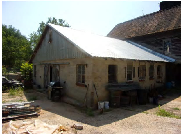
Figure 20. Joseph S. Wells Barn, oblique view of the circa 1960s milk parlor north and west elevations
