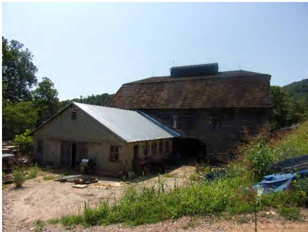
Figure 17. Joseph S. Wells Barn, view to the southeast; the circa 1960s milk parlor is in foreground.
