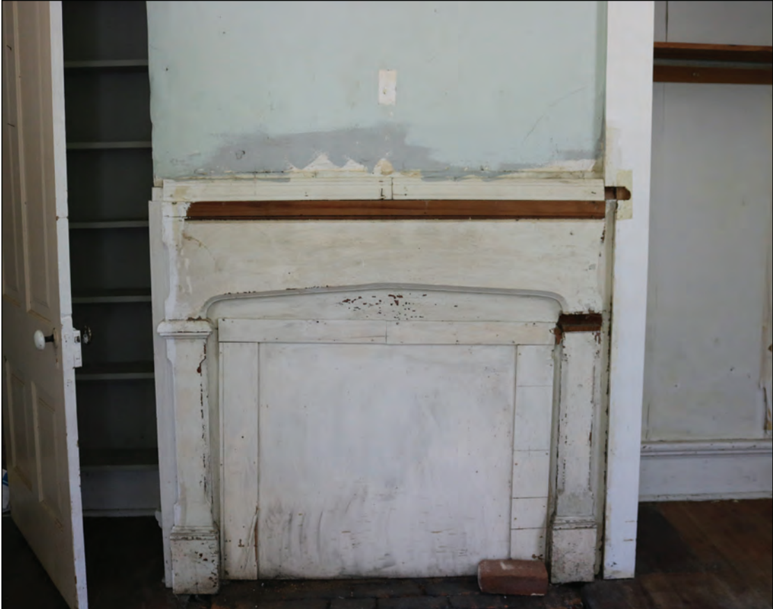
Figure 6.23. Hugh A. Keith House, Mantel and Interior Finishes in the North Room.
