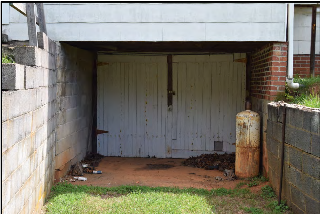
Entrance to lower level garage. The family also kept canned food in the space to preserve it. View to the north
