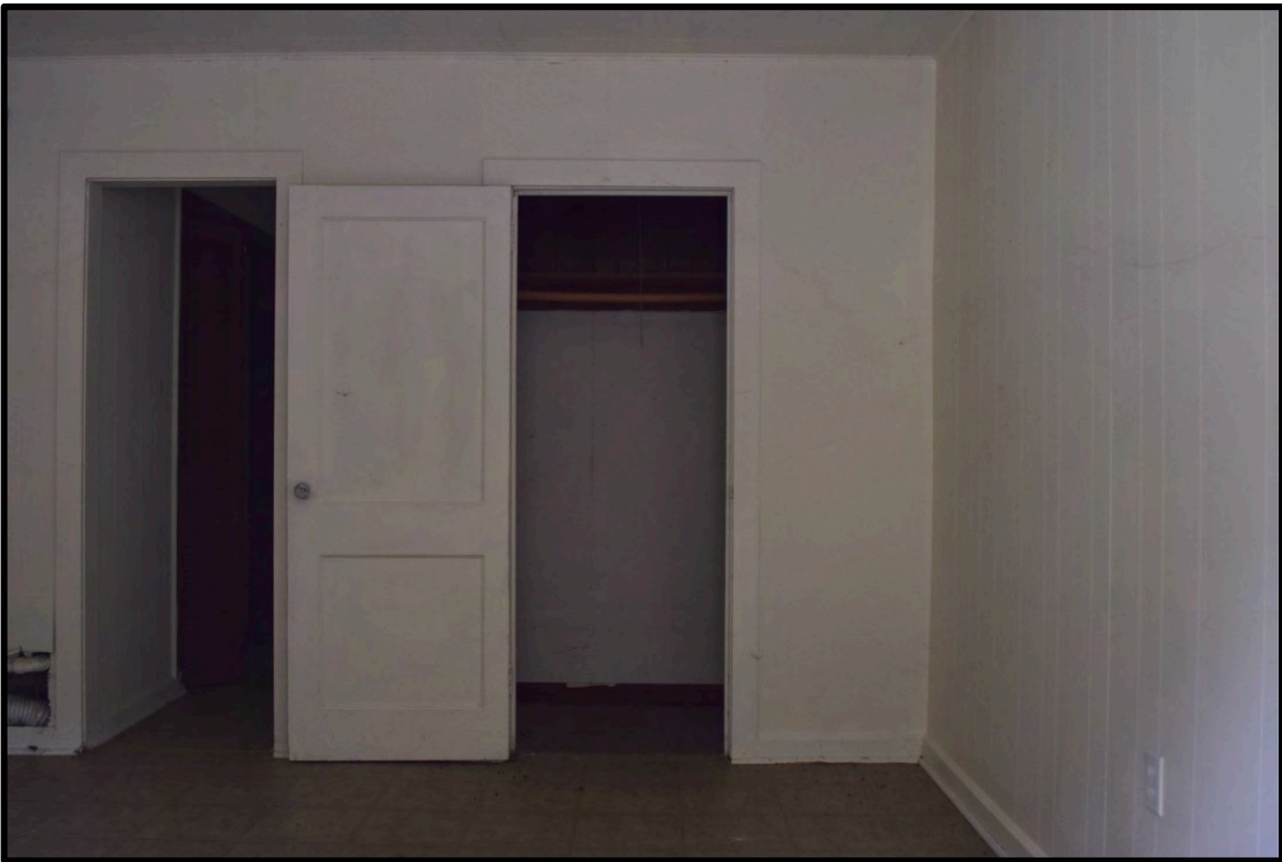
Interior of one of the motor court units, view to the northeast
