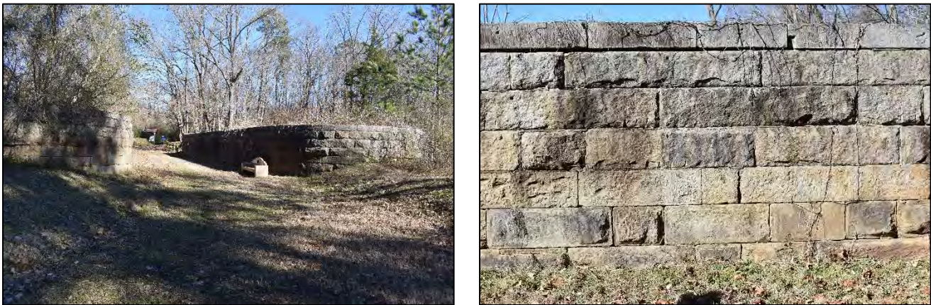
Figure 8. Left, view of approach to aqueduct over creek; right, detail of carefully hewn ashlar blocks
