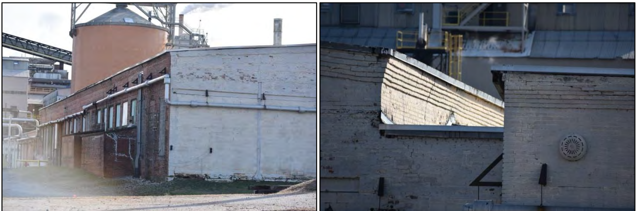
Figure 59. Left, north elevation of paper mill retaining brick wall with altered bays; left, west elevation corbels
