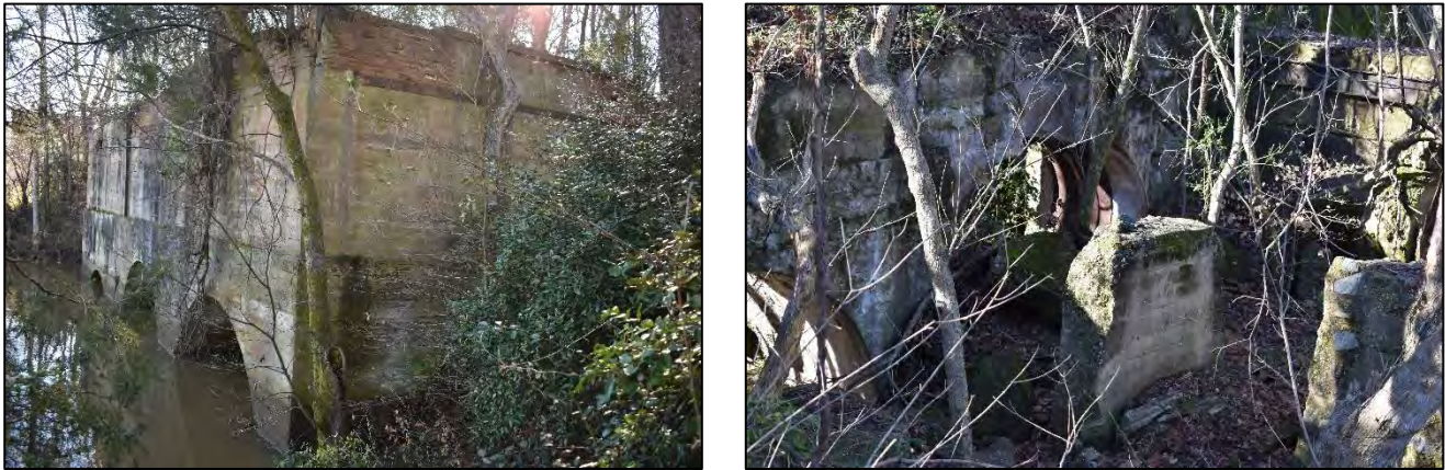
Figure 40. Plant No. 1—left, north and west walls from river edge; right, view with walls
