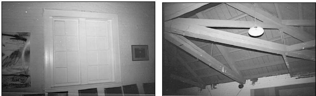
Figure 27. Left, interior view of painted over paired four-over-four sash; right, view of open truss work (photo credit: Allison and David Black)
