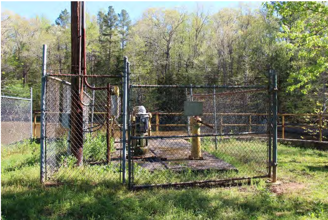
Figure 29. Spillway equipment, view looking northeast.
