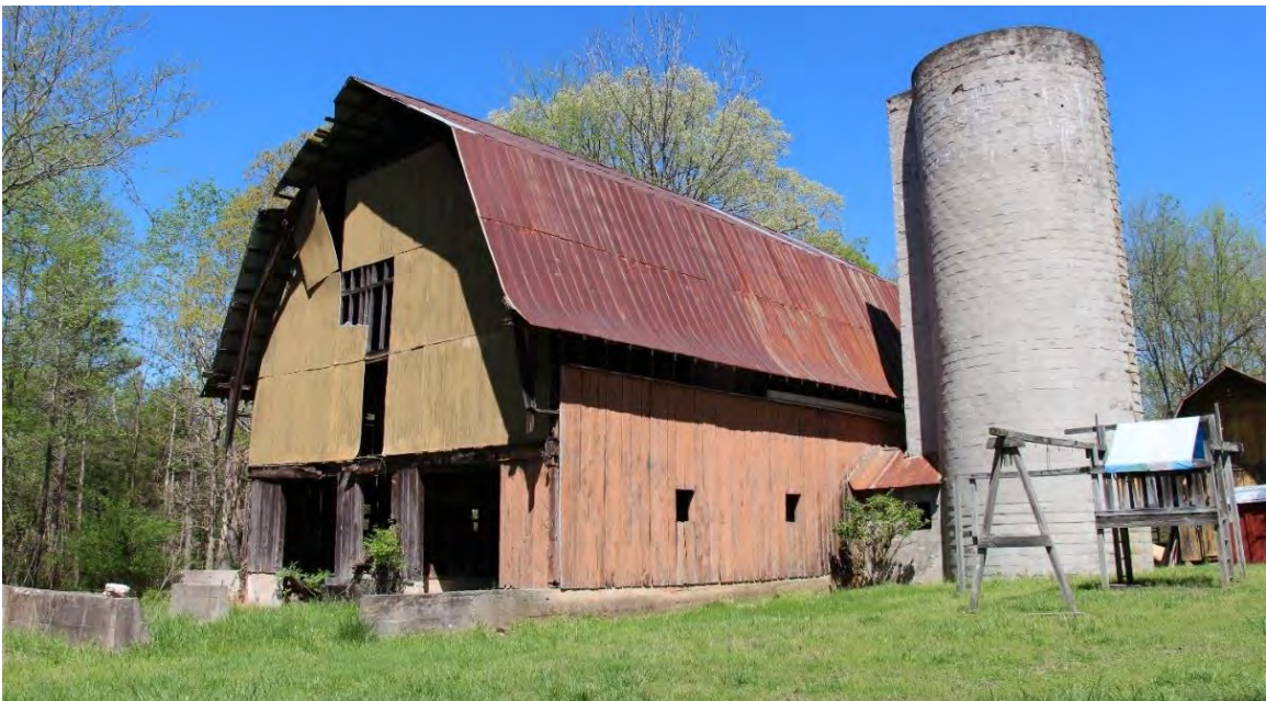
Figure 10. c.1935 livestock/dairy barn and c.1940 concrete silo, facade (south) and side (east) elevation, view facing northwest.
