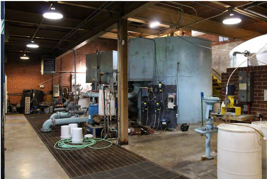
Figure 24. Water tanks (left and center) and alum tank (right).
