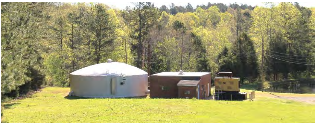
Figure 26. Clear well (left) and pumping station (right), view looking east from water filtration plant catwalk.
