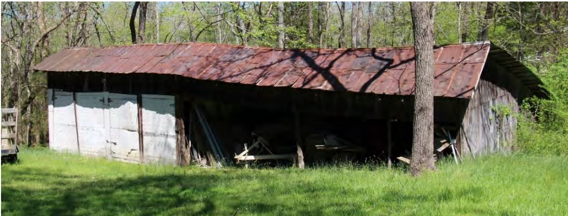
Figure 12. c.1940 equipment shed, facade (south) and side (east) elevation, view facing northwest.
