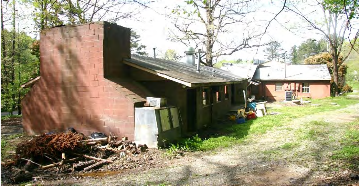
Figure 60. Side (south) elevation of the smokehouse component showing the massive chimney, view looking north.
