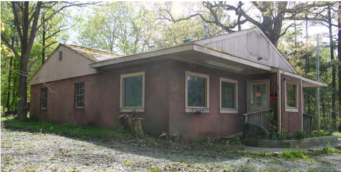
Figure 57. Facade (north) and side (east) elevation of the dining room/kitchen component, view looking northwest.
