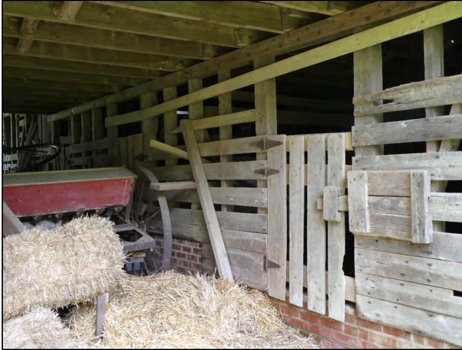
Figure 20. Interior of Transverse-Crib Barn (Site Plan # 3), viewed from western entrance facing southeast.
