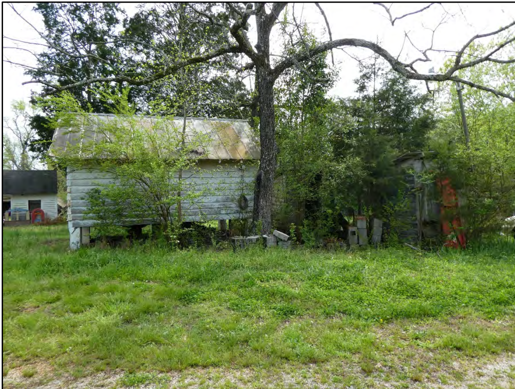
Figure 30. North elevations of Granary A and Privies A & B (Site Plan # 9, 13, and 14), taken facing south-southwest.
