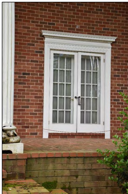
Figure 2.4.4. Julius A. Rousseau House (WK0454), door/window detail, facing south.
