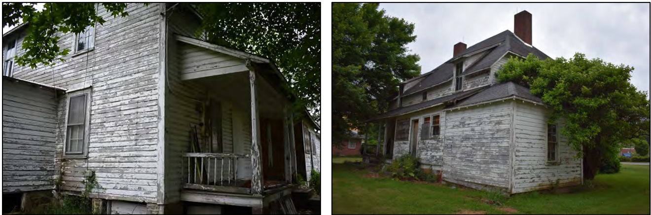
Figure 6. South side and east rear elevations, left; east rear and north side elevations with later-built well house, right
