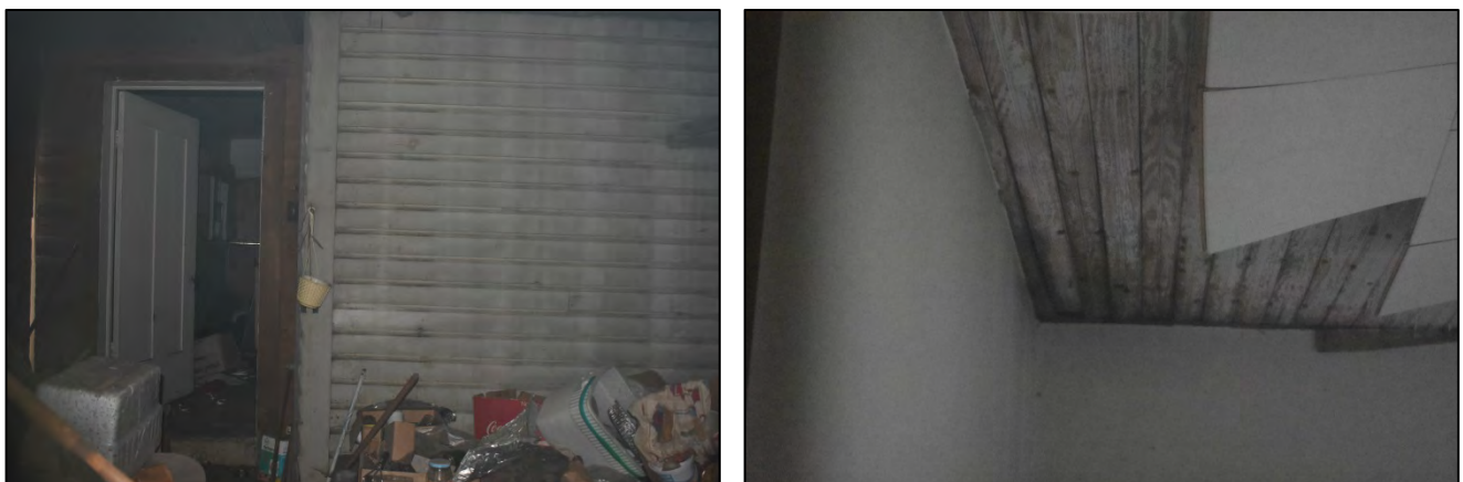
Figure 7. Interior of well house with original northeast corner of house in place and reused two-panel door, left; beaded-board ceiling of sunroom revealed beneath fallen acoustic tiles, right
