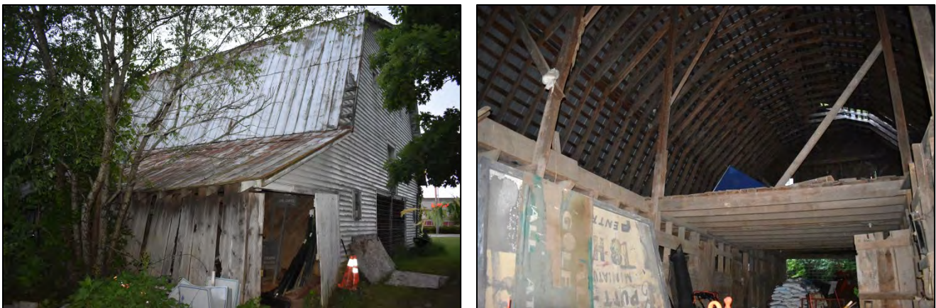
Figure 12. East side and north elevations, at left; stalls, hayloft flooring, and gambrel roof framing, at right
