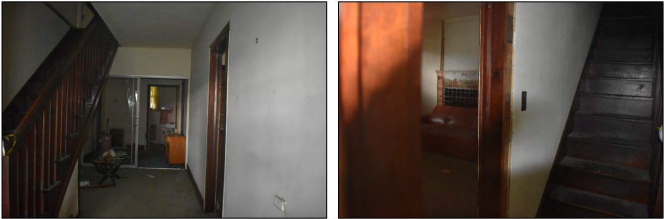
Figure 9. At left, downstairs hall with stair at left, entry into living room at right, and later-added sliding glass door and bathroom at rear; at right, exposed flush boards at entry to, and ghost of mantel in, dining room
