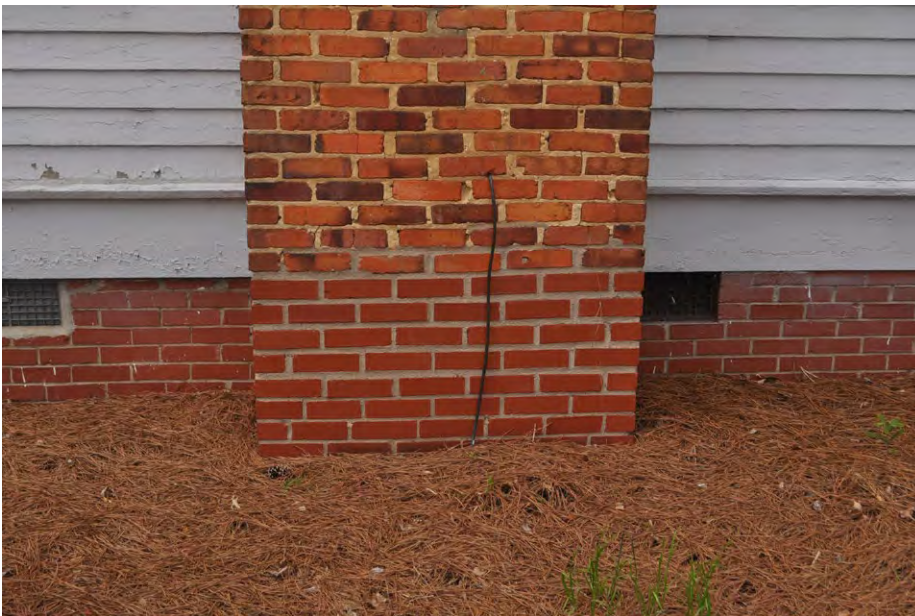
Plate 5.10: View of the base of the chimney on the main block, southeast side of the Moulder House.
