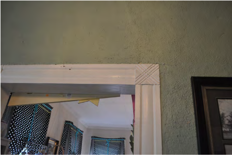
Plate 5.23: View of the southeast front room, first floor, and the door trim.
