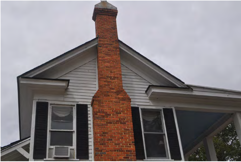
Plate 5.13: View of the gable end return of the southeast main block of the Moulder House.
