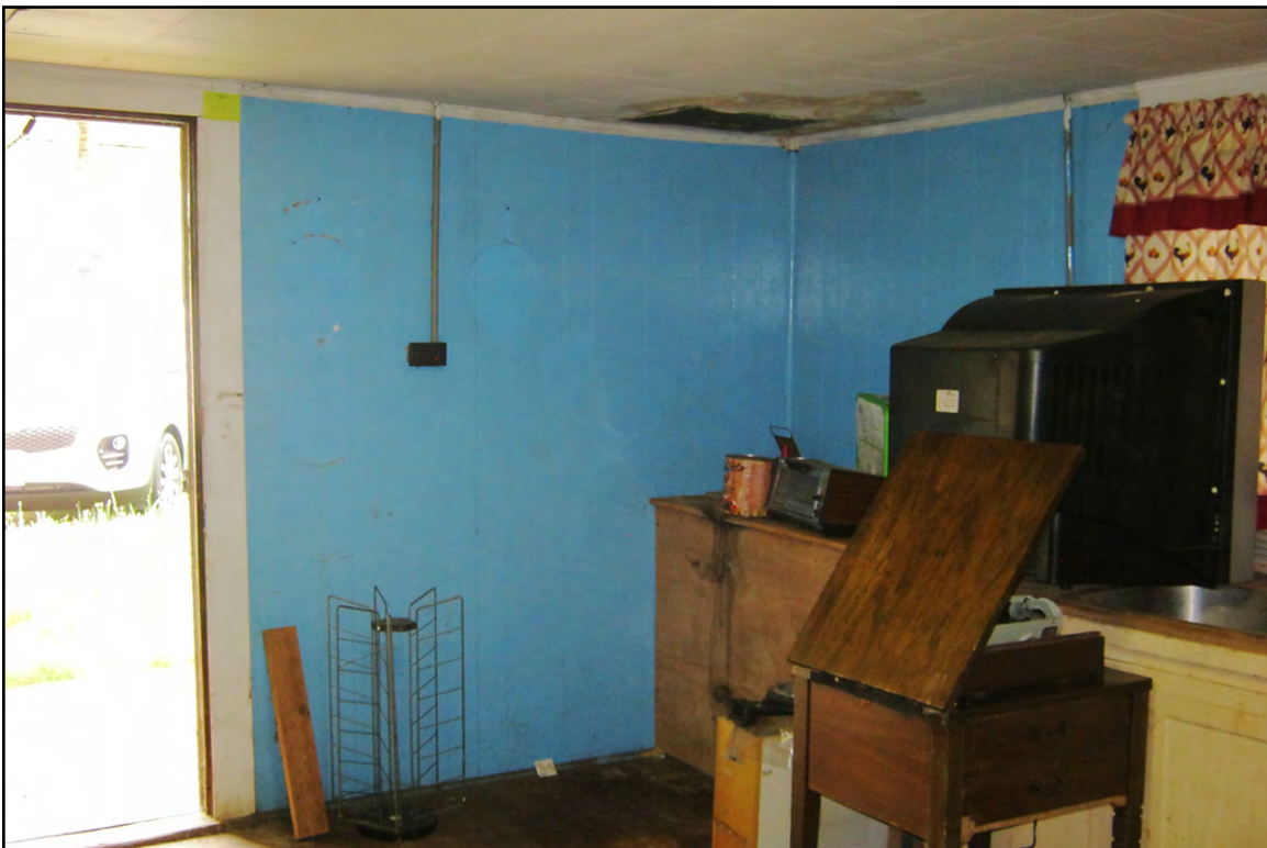
PLATE 9: Former Gulf Gas Station (RK1128), Interior View of Kitchen, Rockingham County, North Carolina
