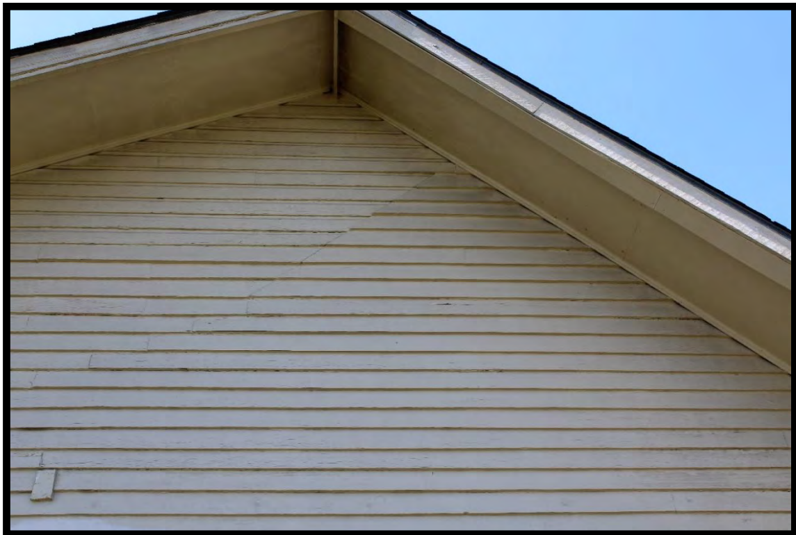
Figure 48: Giles Stephens Homeplace, Detail of East Elevation Showing Ghost Mark of Lower Gable. Note change in siding from plain weatherboard to German lap siding.
