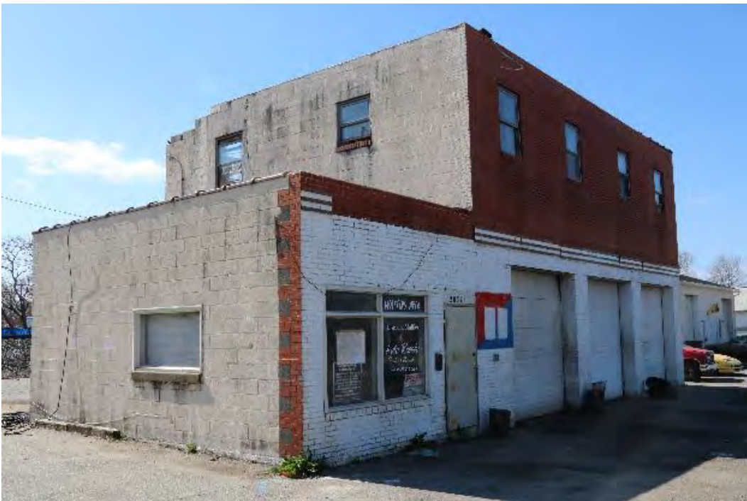
Figure 11. Front (north) and side (east) elevation, view facing southwest. Mead & Hunt photograph.
