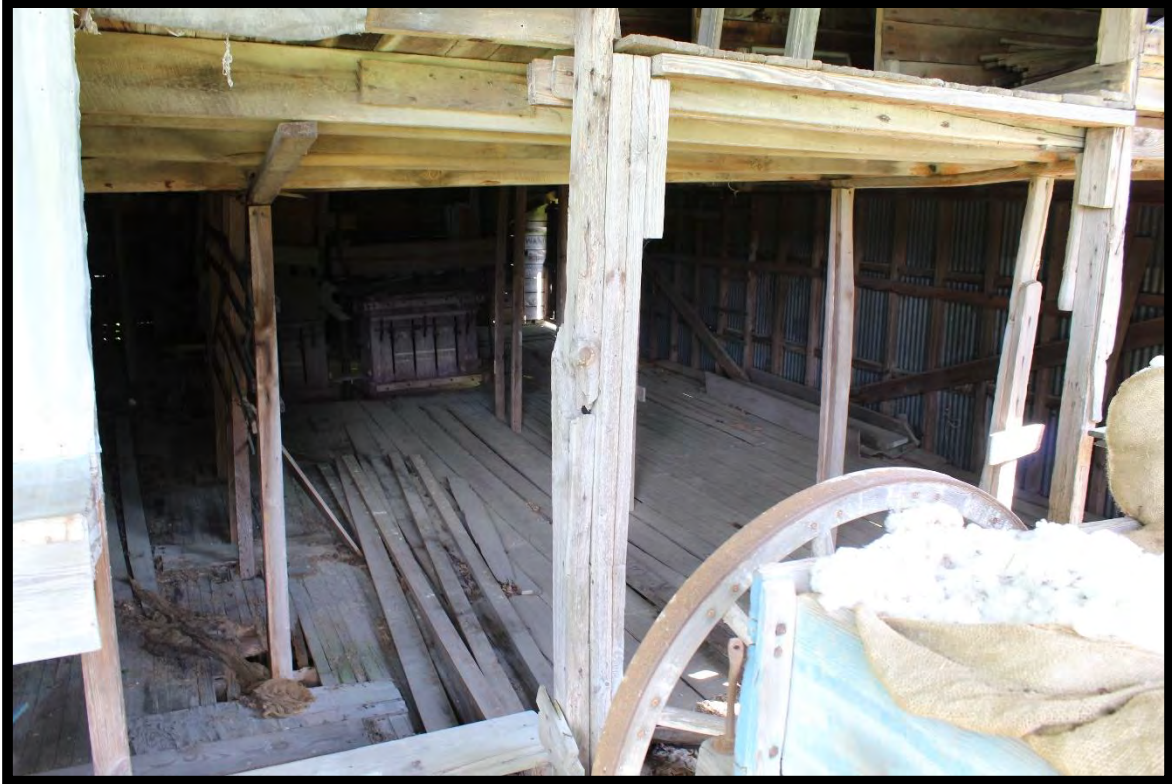
Figure 40: Gillis Cotton Gin 2, View of Ground Floor and Drive Shafts, Looking Southeast.
