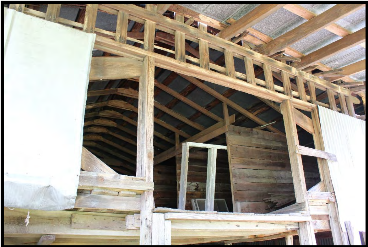
Figure 41: Gillis Cotton Gin 2, View of Divided loft in upper story, Looking Southeast.
