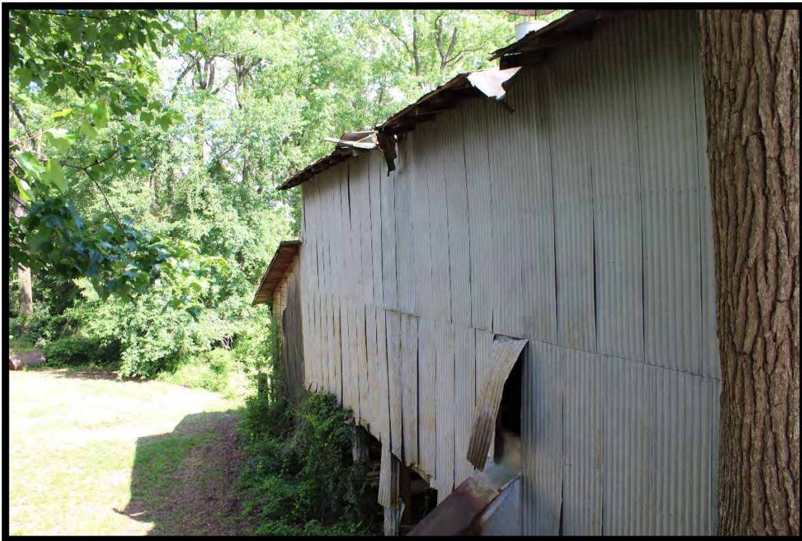
Figure 39: Gillis Cotton Gin 2, View of Side Elevation and Seed House, Looking Southeast.
