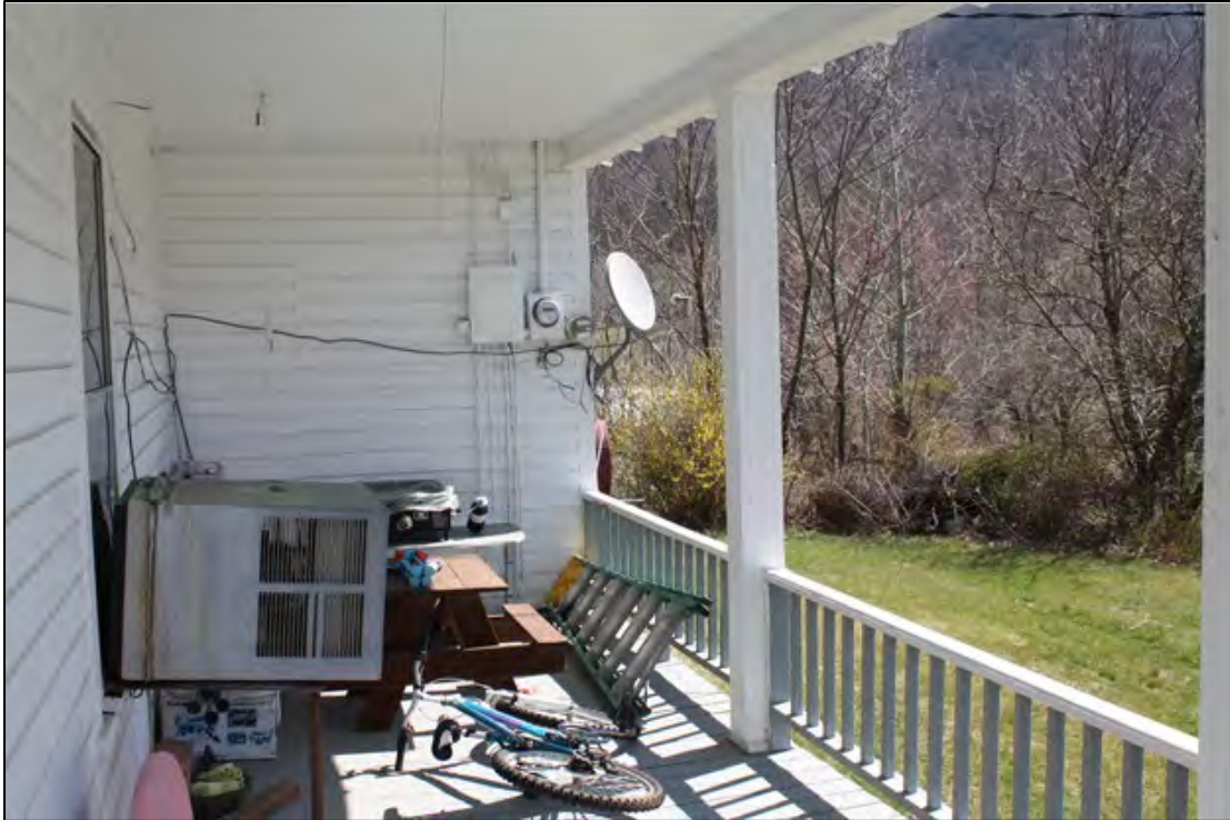
Figure 5: Looking north on the front porch. An area of patched siding can be seen on the far wall where a door was once present.
