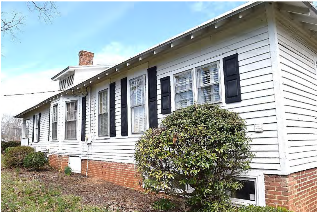
Plyler Family Homeplace, Main Block and Rear Ell, Side (South) Elevation, Replacement Windows, Looking Northwest.
