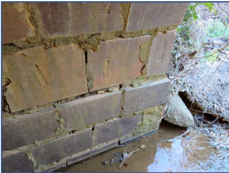
Arch Culvert (Pipe #40 2112) SR 2735 (Sockwell Road) Guilford County Looking south (above). Detail of segmental and rectangular Pomona block at south end (below). Photographed 13 January 2016.
