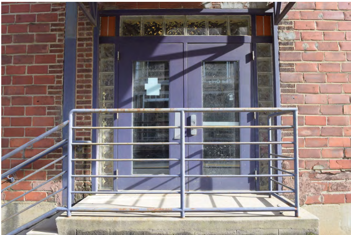
Modern doors on northwest elevation of the north building along Meadow Road, view to the southeast
