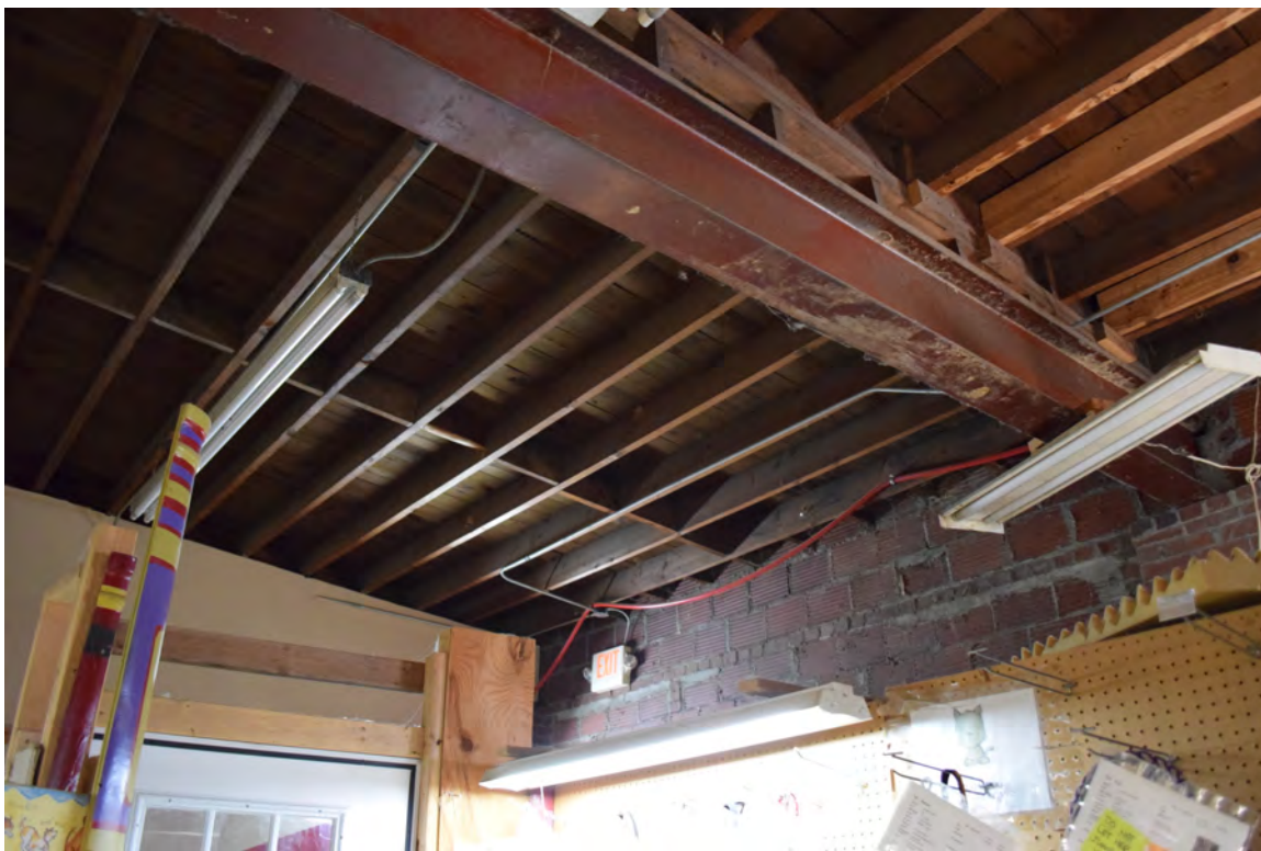
Intact interior finishes and structural elements including steel I-beams remain intact in the warehouse
