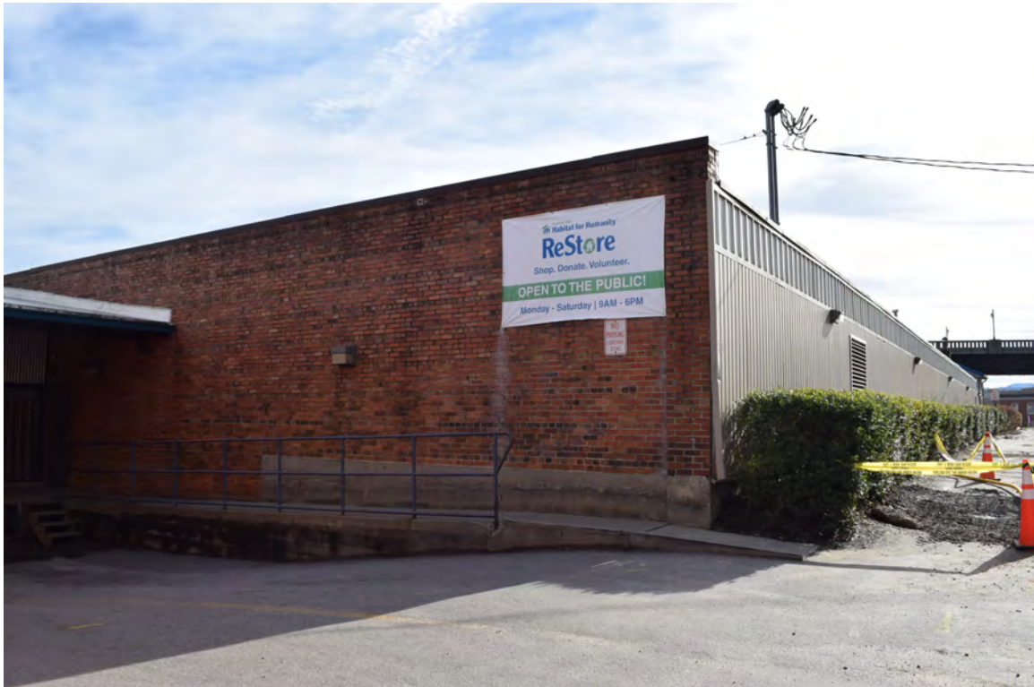
North wall of southern warehouse with brick exposed, view to the southwest
