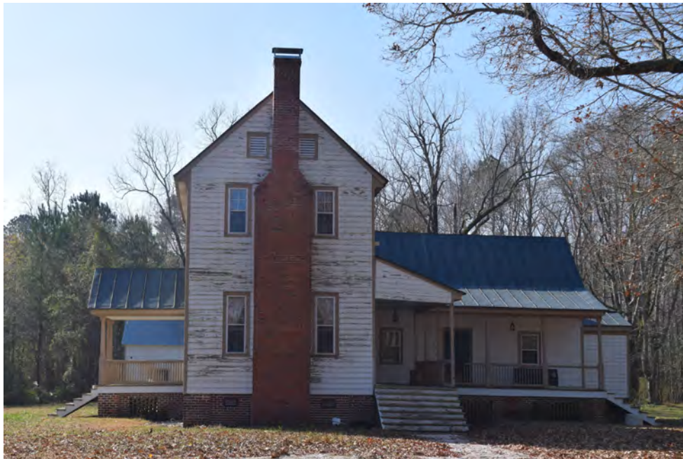
North elevation of the King-Freeman-Speight House (BR0098, NR), view to the south
