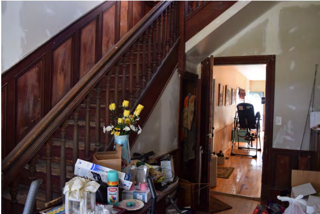
Central passage of main block looking into rear ell, view to the west southwest
