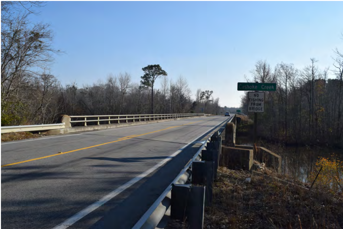
Bridge over Cashoke Creek built in 1967 near the south end of the project area, view to the south
