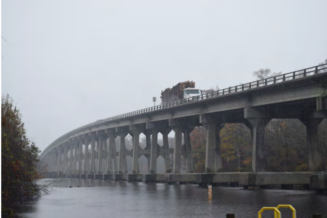
Bridge over the Roanoke River at the south end of the APE, view the northeast
